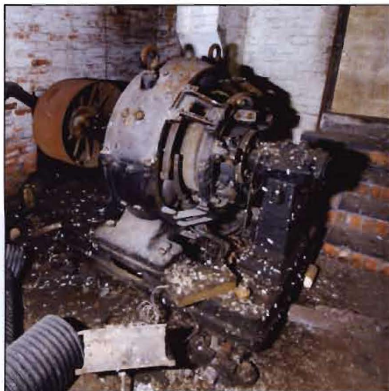
Figure 52. One of the 1922 DC electric motors in the Motor Room. [DP043927]
