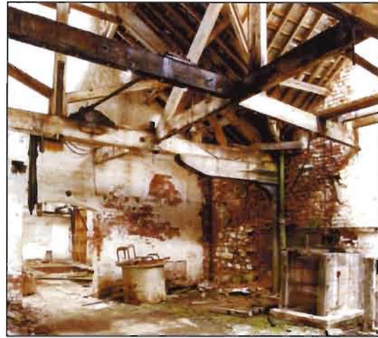
Figure 45. Heavily-built ventilated roofs and multiple phases of wall construction in the eastern part of the Dye Works. [AA96/00711]
