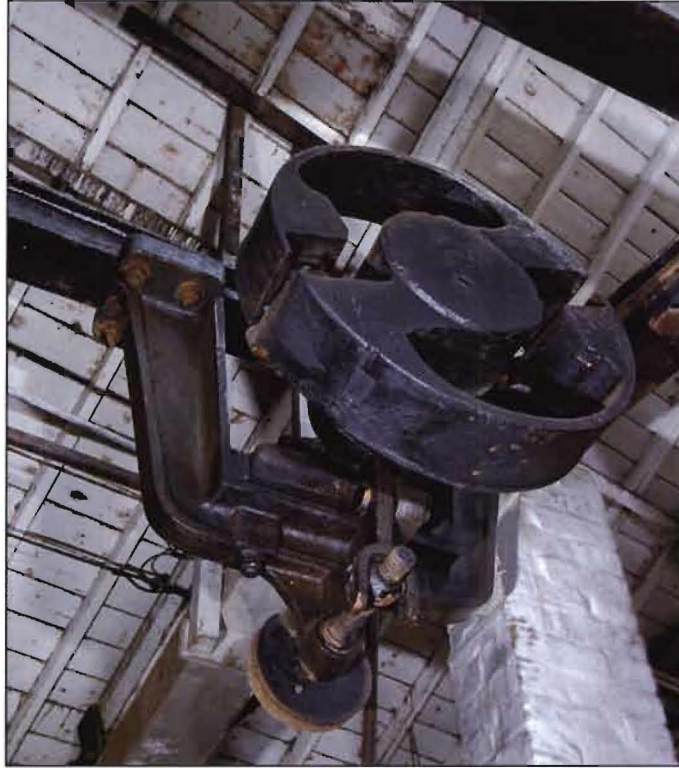
Figure 42. The friction clutch is still attached to the water-powered shaft above the wheel chamber. [DP043906]
