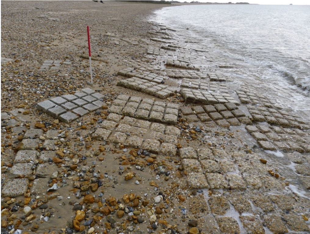
Figure 45. Disturbed areas of 'chocolate block' concrete matting at embarkation hard G1, view to east, scale 1m (© Historic England, photograph by Wayne Cocroft).
