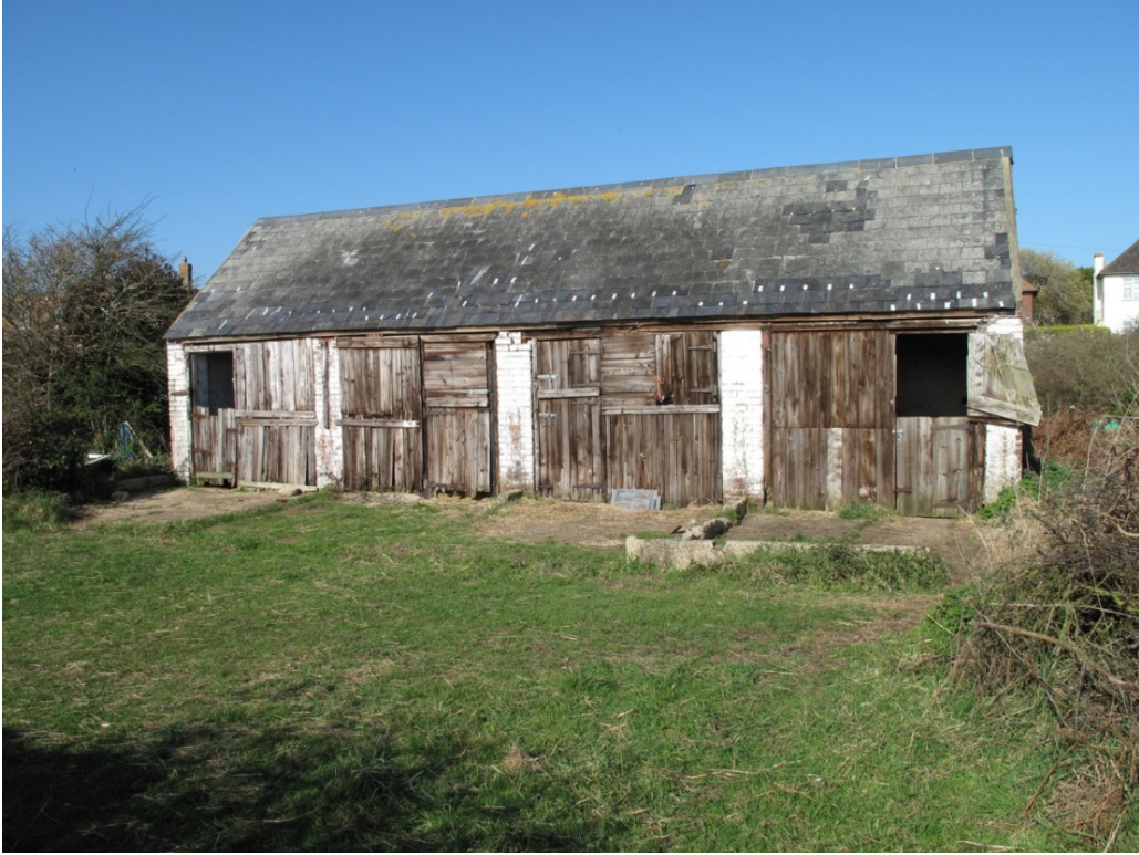
Figure 30. Southern elevation of brick building on the northern edge of Battery 4 (© Historic England).
