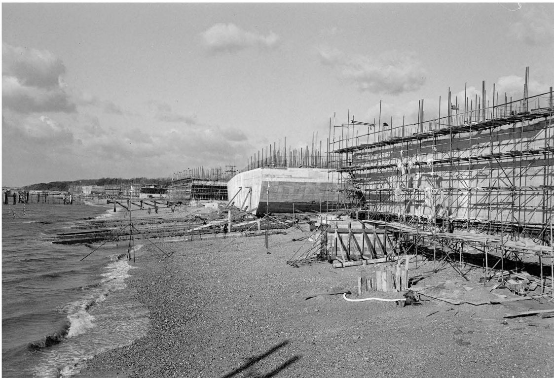
Figure 9. Phoenix caissons under construction at Stokes Bay, 1944 (copyright Imperial War Museum, H 35554).
