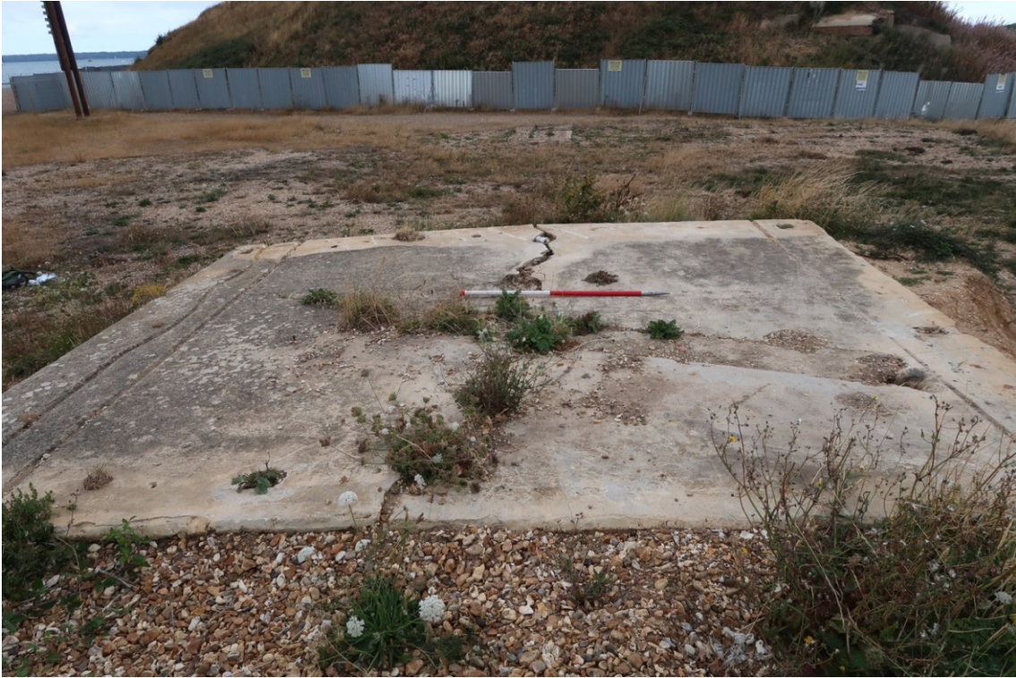
Figure 72. Concrete base for search light position 1, looking west towards Fort Gilkicker, scale 1m (© Historic England).
