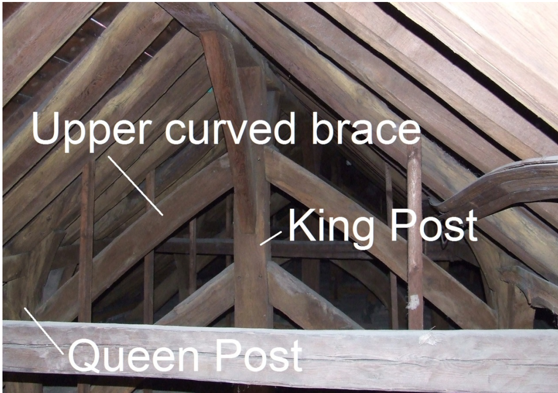
Figure 2: View of a roof truss showing the unusual combination of king post, queen post, and curved struts (photograph Martin Bridge)
