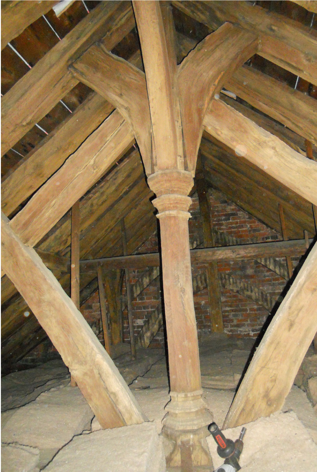
Figure 3: View of the decorated crown post at the southern end of the roof (photograph Martin Bridge)
