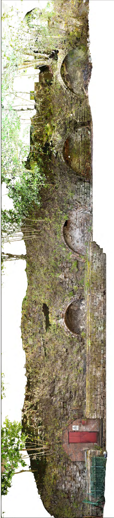
Fig 51. The five alcoves along the rear wall of the Heritage Railway yard, corresponding to the former location of the blast furnaces. The images is derived from a laser/orthophotographic scan taken in 2018 to inform conservation measures. © Historic England.
