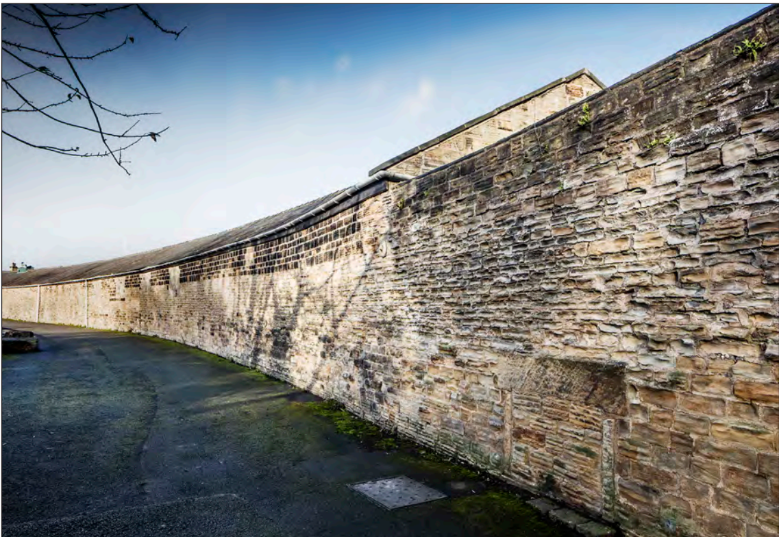
Fig 83. (a) above: Building 4-7A, north-east elevation, L Jessop, June 2017 and (b) below: Building 4 and 5 from Forge Lane, Alun Bull, October 2017. © Historic England.
