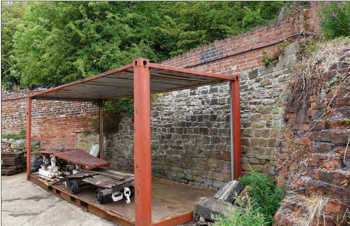
Fig 56. The northern section of ironworks/Heritage Railway yard wall, incorporating reused brick and earlier in-situ masonry, D Went, August 2018 © Historic England.
