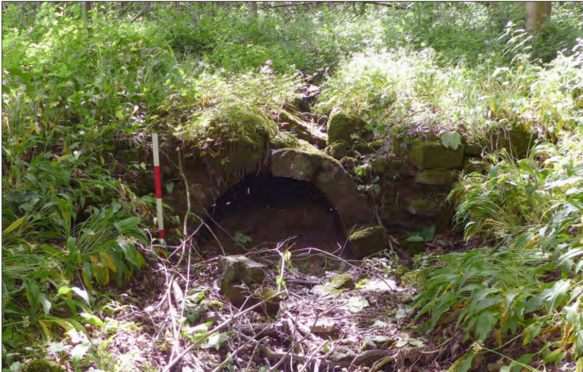
Fig 93. The culvert forming the main sluice from the Linthwaite reservoir – a tunnel of un-frosted brick, typical of the late 19th century, faced with a sandstone arch, D Went, June 2017. © Historic England.
