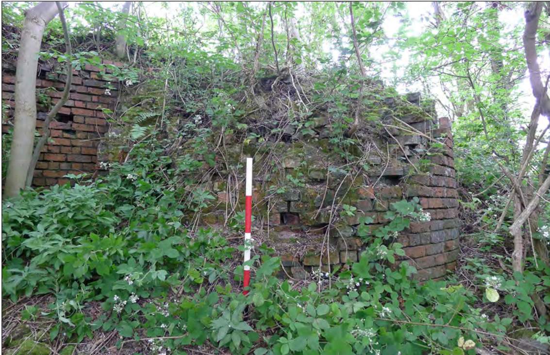
Fig 57. The chimney base to the south of the boiler yard which is shown on the 1859 plan, D Went, June 2017 © Historic England.
