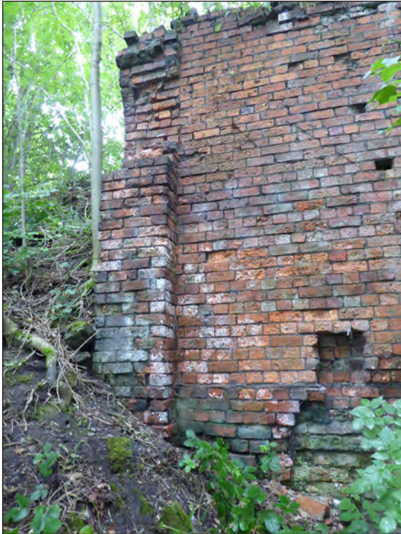
Fig 61. The south entrance to the blowing engine house viewed from within (P1000757). Note the short return with traces of the arch above, and the iron plate set within the lower brick courses, J Rimmer, July 2017. © Historic England.
