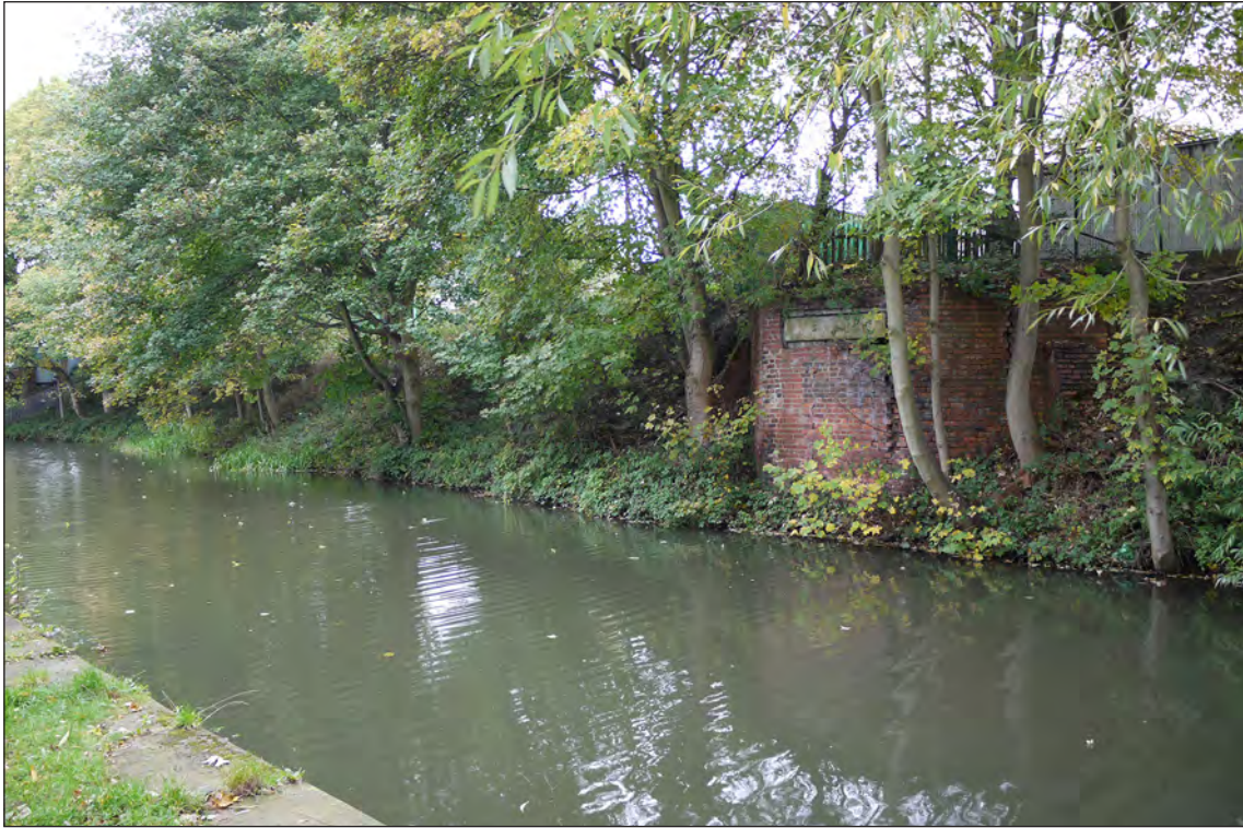
Fig 96. Simon Wood footbridge abutment and the masonry landing, D Went, October 2017. © Historic England.
