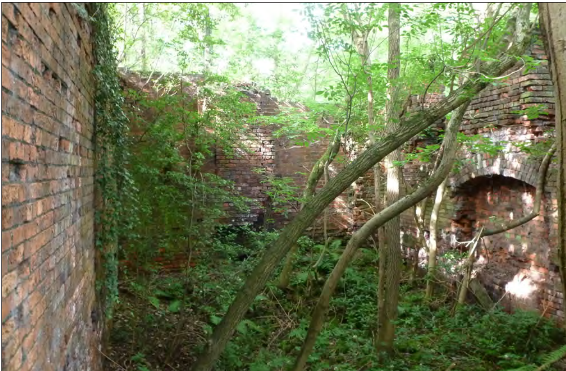
Fig 60. The interior of the blowing engine house facing south. Note, behind the trees, the blocked door (right) and window (left) apertures in the south wall. The declivity across the interior ground surface is also visible, J Rimmer, July 2017. © Historic England.
