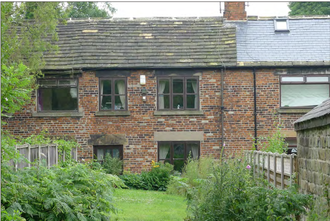
Fig 89. (a) above: Nos. 9-11 Distillery Side from the front and (b) below: 11 Distillery Side from the rear, L Jessop, June 2017. © Historic England.
