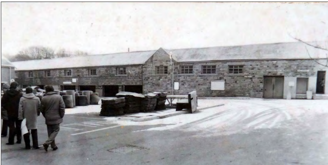
Fig 84. (a) Building 5, north-east elevation ground-floor openings supported on iron columns and plates (now blocked), L Jessop, June 2017. © Historic England; (b) 1980s photograph of the Forge Lane range, reproduced with kind permission of Barnsley Archives and Local Studies, NCB workshops archive photo 8.
