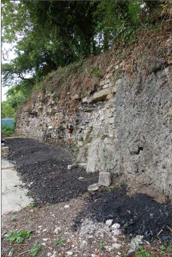
Fig 54. Part of the retaining wall to the rear of the Elsecar ironworks, viewed from the south. Note the projecting sandstone ‘throughs’ which indicate the depth of masonry facing which has otherwise been stripped away, and the water-borne deposits coating and projecting from the wall in the foreground, J Jenkinson, August 2018 © Historic England.
