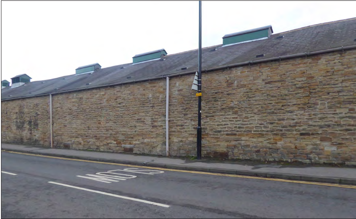
Fig 82. Wath Road range, showing sooting (far left of frame) and ventilation grilles (at ground level) to Building 11, J Rimmer, December 2018. © Historic England.
