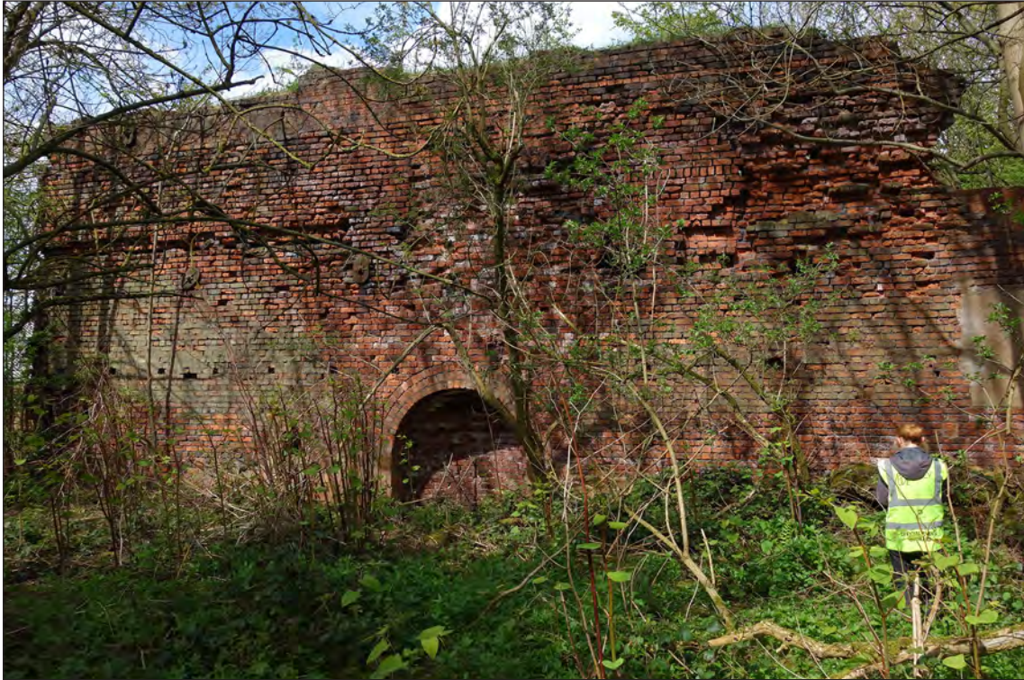
Fig 58. The south wall of the narrow passage-like building across the northern side of the former boiler yard. Note the springing for the yard archway, and the curious alcove at the base of the elevation. D Went, January 2017 © Historic England.
