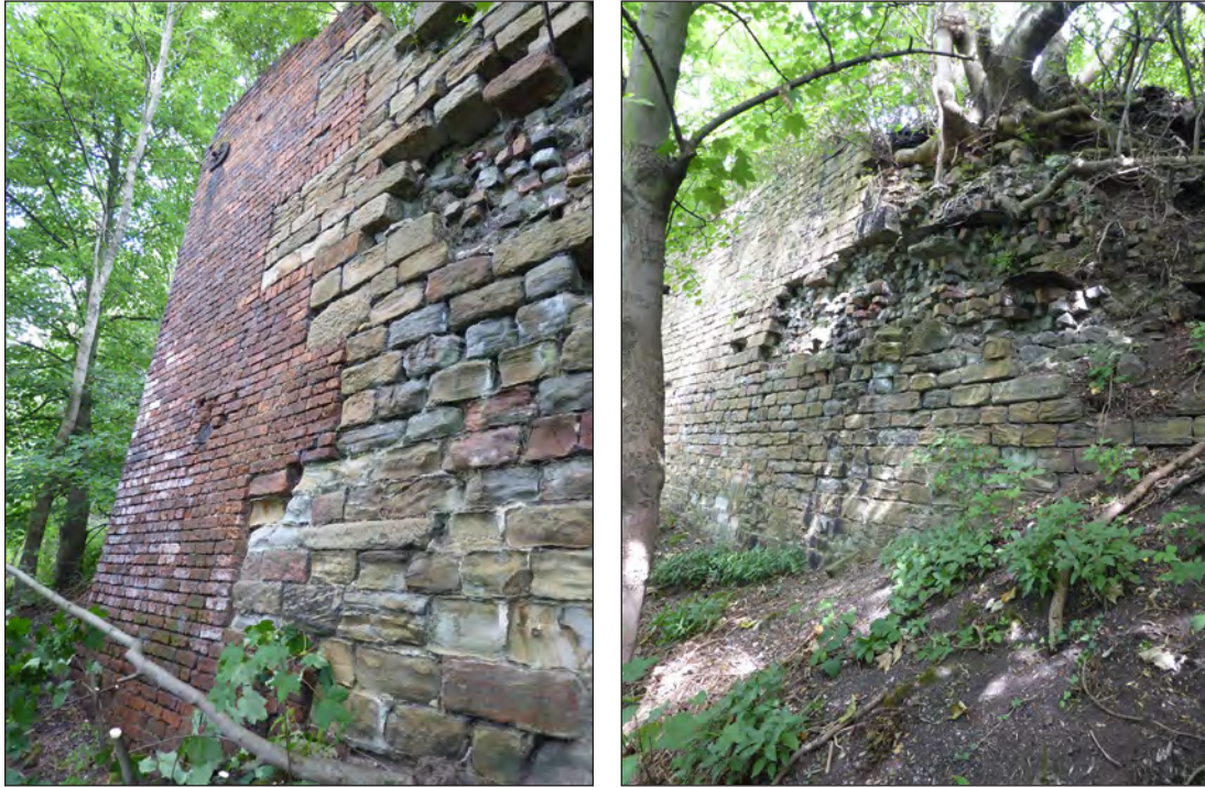
Fig 50. (a) North corner of the furnace bank wall, showing the transition from stone to brick and part of the exposed rubble core, and (b) the southern end of the remaining furnace bank wall. J Rimmer, July 2017. © Historic England.
