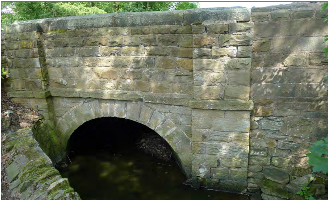
Fig 108. Road bridge over the Harley Dike, Wentworth Road, L Jessop, July 2017 (P1240157). © Historic England.
