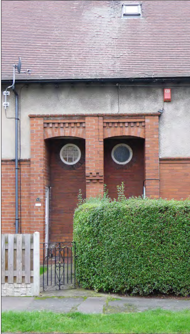
Fig 191. (a) Nos. 41-45 Strafford Avenue, detail of internal porches and (b) Nos. 11-17 Cobcar Avenue, D Went, October 2017. © Historic England.
