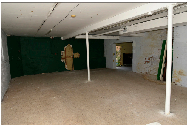
Figure 29: The row of cast iron columns and timber beam which carried the first floor over the ground floor store of the main range. © Ark Property Services
