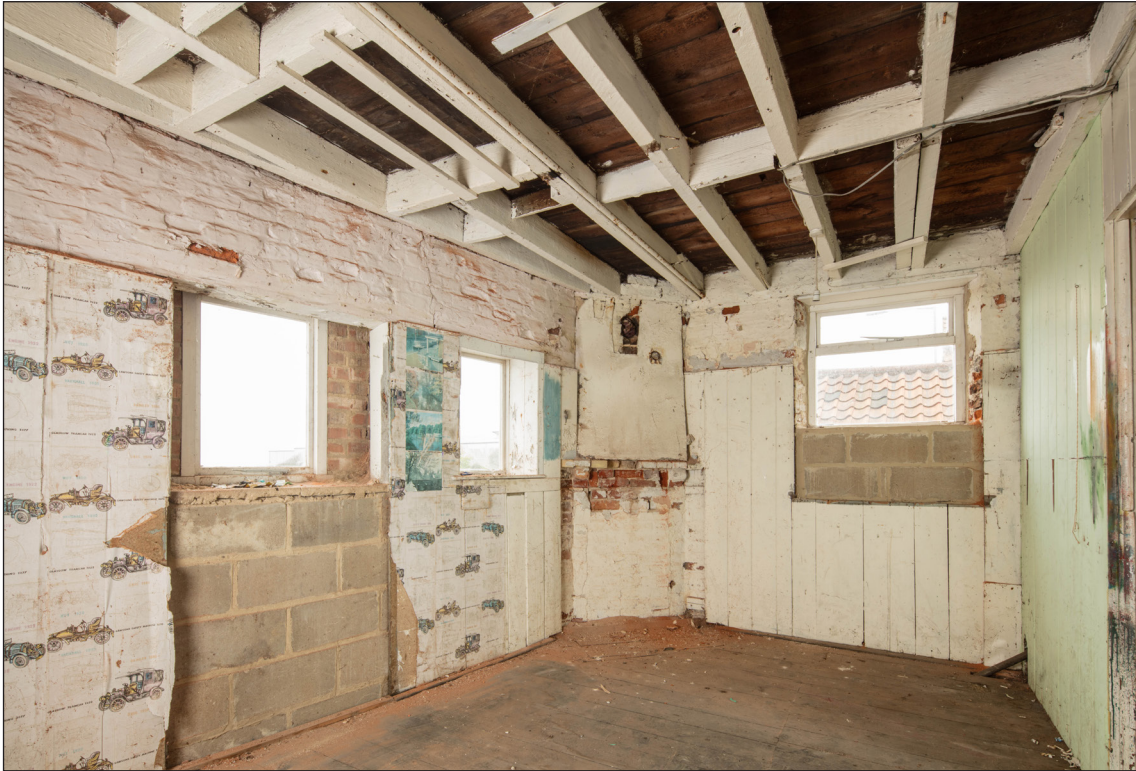
Figure 58: The office created at the eastern end of the first floor which dates from the building's use as a holiday hire business. © Historic England, Patricia Payne, DP247707
