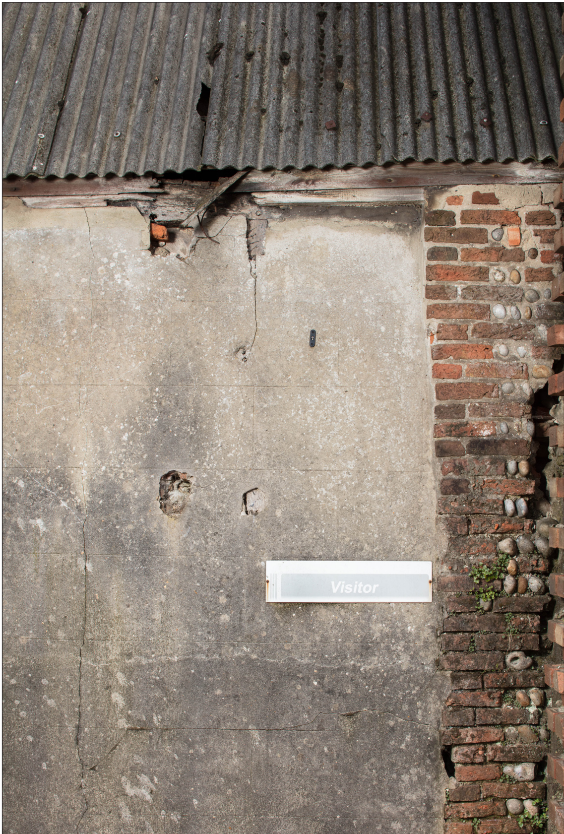
Figure 38: Part of the northern elevation of the northern range of 315 Whapload Road showing the joints between the different phases of fabric and the cracked render revealing a timber frame. © Historic England, Patricia Payne, DP247731
