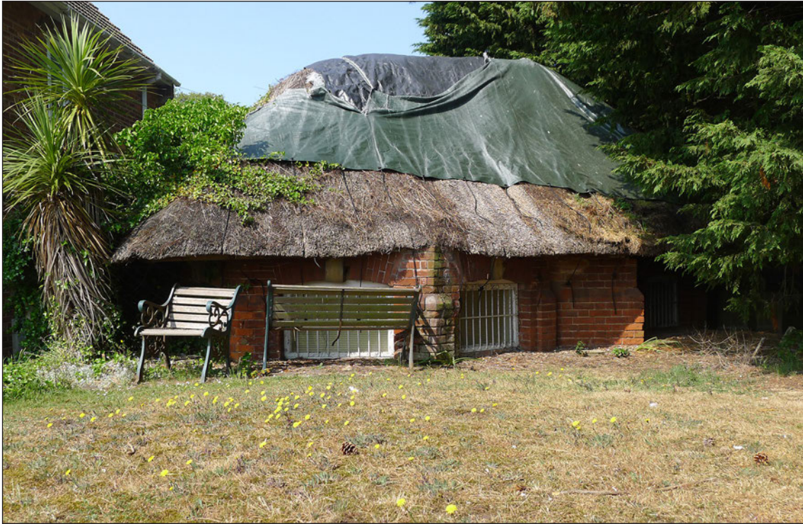
Figure 50 – The garden building that is thought to have been adapted as a shell store for the Gunton Battery (Magnus Alexander, with permission, © Historic England)
