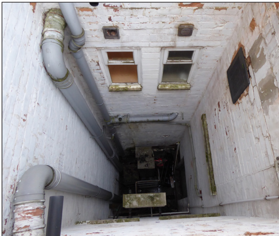
Figure 13: View looking down the light well at the rear of the property (© Historic England, photograph: Alastair Coey Architects 2019)
