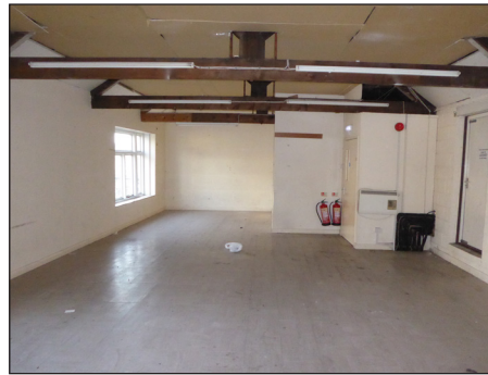
Figure 27: (a) Interior of the second-floor storage space with exposed trusses (© Historic England, photograph: Alastair Coey Architects 2019)
