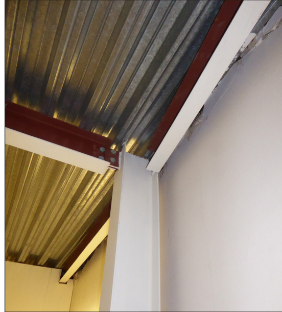
Figure 16: The internal steelwork structure on the ground floor (© Historic England, photograph: Alastair Coey Architects 2019)
