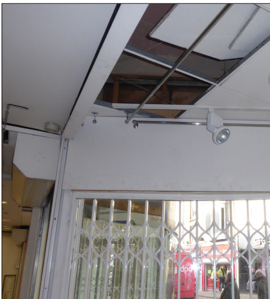
Figure 21: Detail of removed ceiling panels in shop display units showing blocked window openings above transom level (© Historic England, photograph: Alastair Coey Architects 2019)
