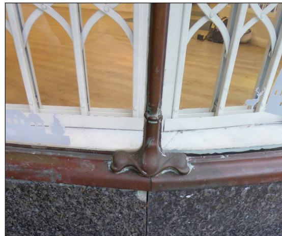
Figure 11: Art Nouveau bronze details on the shopfront (© Historic England, photograph: Alastair Coey Architects 2019)
