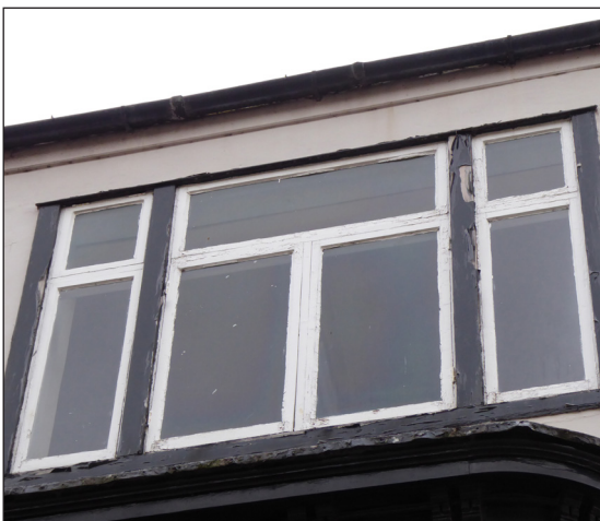
Figure 25: (a) External view of the second-floor windows (© Historic England, photograph: Alastair Coey Architects 2019)
