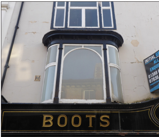
Figure 24: (a) External view of the first-floor oriel windows (© Historic England, photograph: Alastair Coey Architects 2019)
