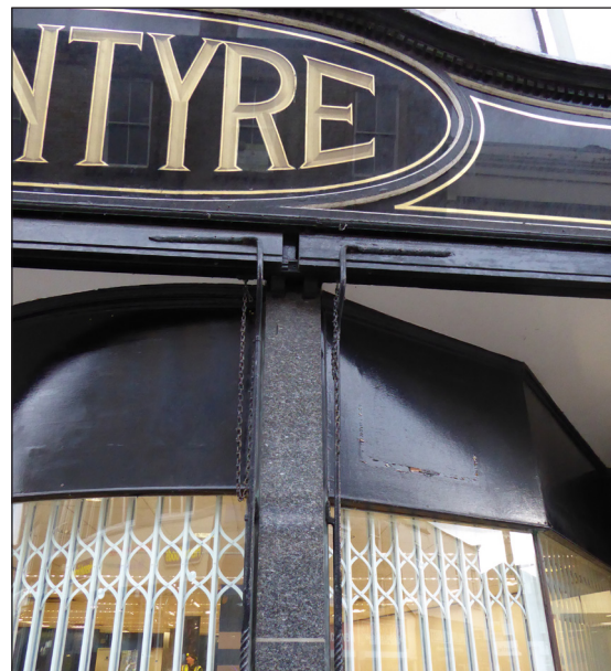
Figure 22: Detail of arms for the concealed awning (© Historic England, photograph: Alastair Coey Architects 2019)
