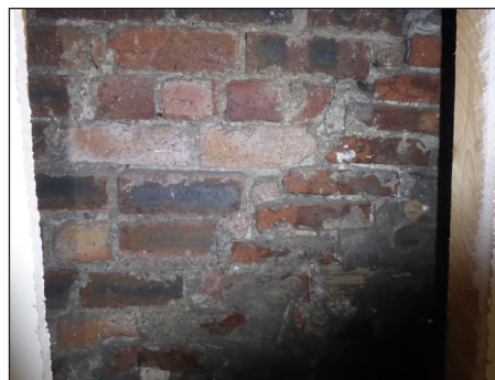
Figure 28: Detail of brickwork in south gable wall (© Historic England, photograph: Alastair Coey Architects 2019)
