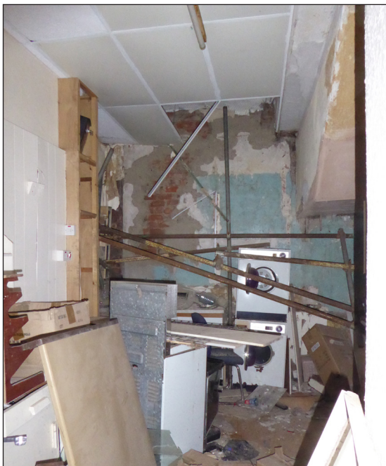
Figure 39: View of the ground-floor rear room (© Historic England, photograph: Alastair Coey Architects 2019)
