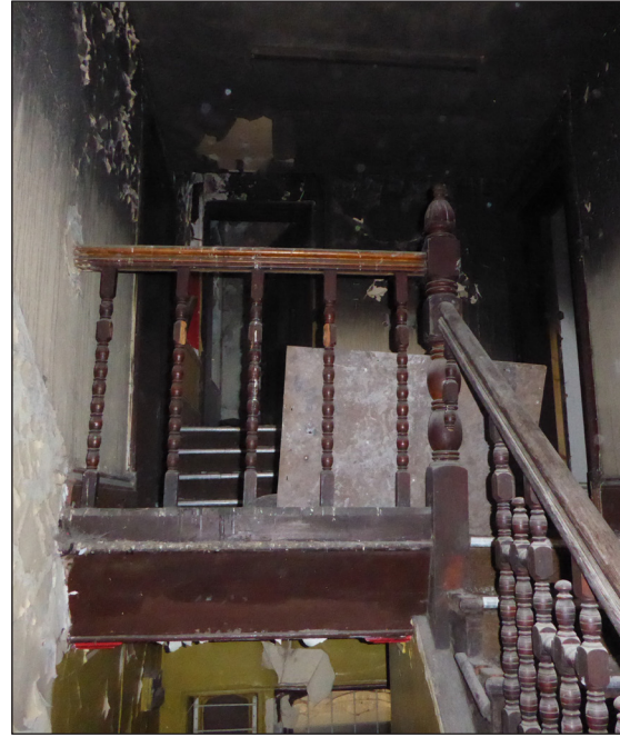
Figure 38: The first-floor landing with the altered stairs continuing to the second floor in the extension behind (© Historic England, photograph: Alastair Coey Architects 2019)
