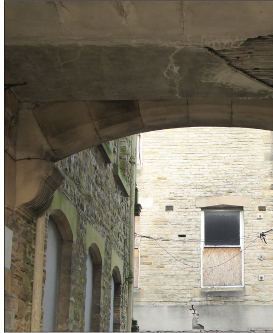
Figure 28: Detail of the brackets on the underside of the bridge (© Historic England, photograph: Alastair Coey Architects 2019)
