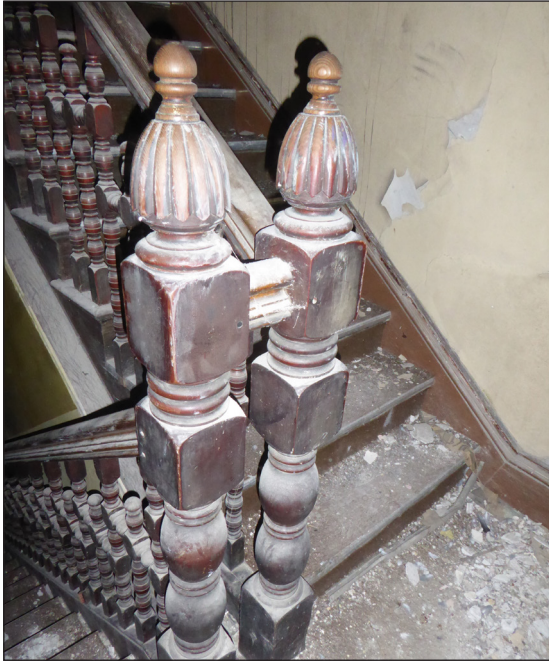
Figure 37: Detail of newel posts on the mezzanine landing (© Historic England, photograph: Alastair Coey Architects 2019)
