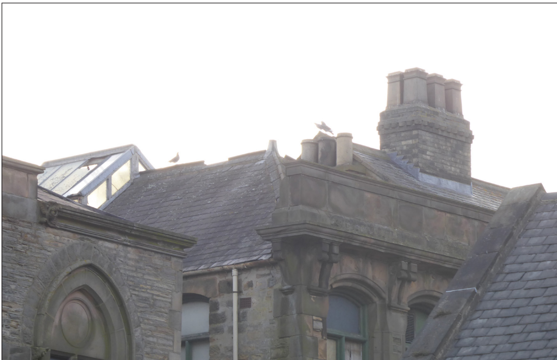
Figure 32: Detail of the parapet and roof lantern of the Mechanics' Institute (© Historic England, photograph: Alastair Coey Architects 2019)
