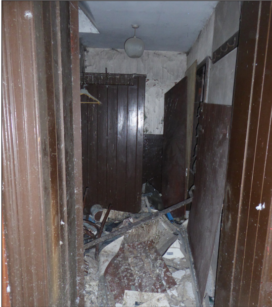
Figure 58: View into second-floor toilets and cloak room lobby (© Historic England, photograph: Alastair Coey Architects 2019)
