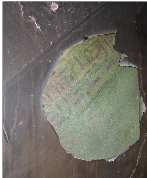
Figure 50: Detail of stencilled geometric wall decoration on second-floor staircase (© Historic England, photograph: Alastair Coey Architects 2019)
