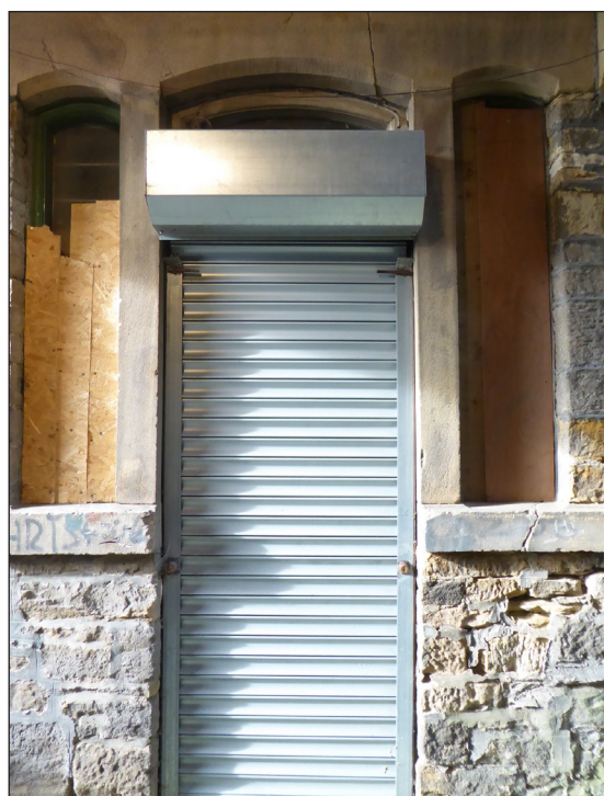
Figure 25: Secondary (alleyway) entrance of the Mechanics' Institute (© Historic England, photograph: Alastair Coey Architects 2019)
