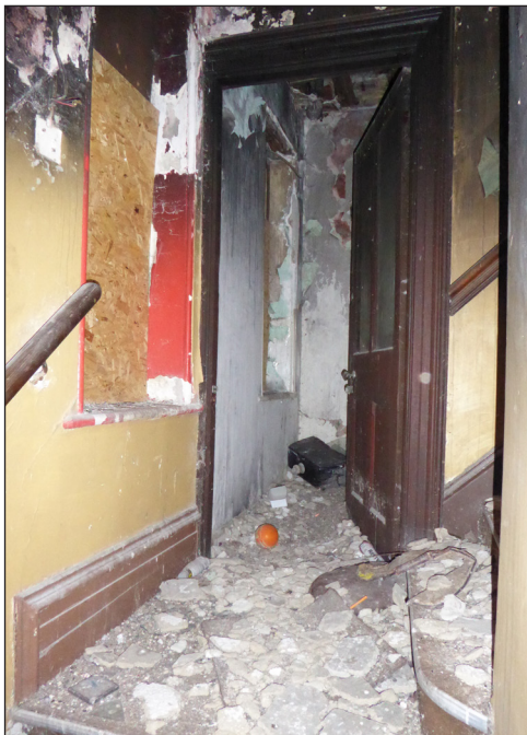
Figure 47: View of first-floor alleyway bridge landing looking into the small room to east (© Historic England, photograph: Alastair Coey Architects 2019)
