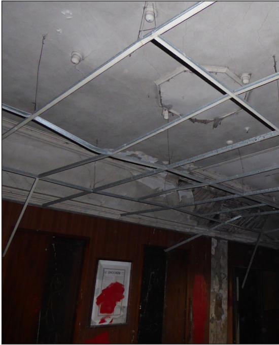
Figure 53: View of second-floor ceiling above 20th-century suspended ceiling (© Historic England, photograph: Alastair Coey Architects 2019)
