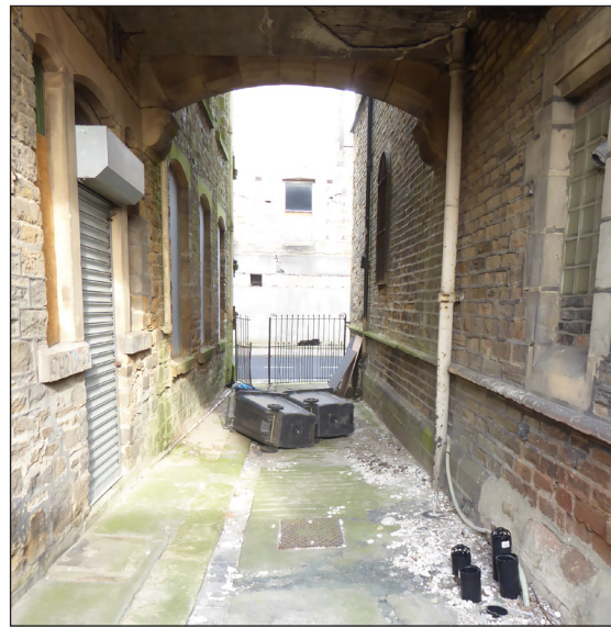
Figure 14: The passageway to the east of the Mechanics' Institute building (© Historic England, photograph: Alastair Coey Architects 2019)
