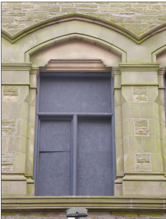
Figure 22: Second-floor window of the Mechanics' Institute (© Historic England, photograph: Alastair Coey Architects 2019)
