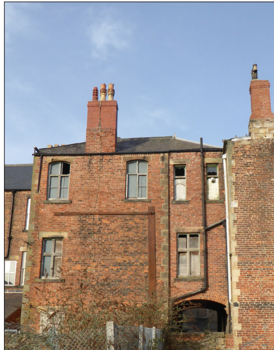
Figure 30: Rear elevation of the Mechanics' Institute from the brownfield site to the south (© Historic England, photograph: Alastair Coey Architects 2019)
