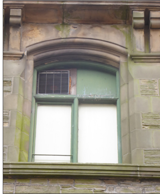
Figure 52: External view of central second-floor window and vent (© Historic England, photograph: Alastair Coey Architects 2019)
