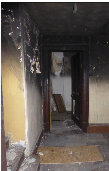
Figure 44: View of first-floor landing looking to the rear rooms (© Historic England, photograph: Alastair Coey Architects 2019)
