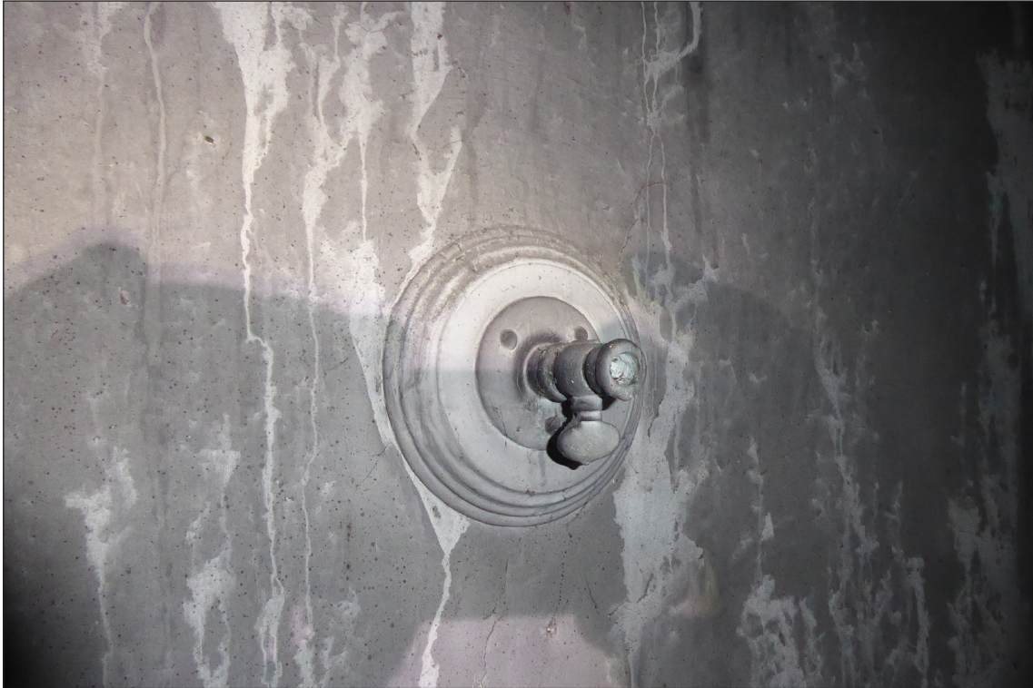
Figure 48: Detail of gas sconce in small room in archway bridge (© Historic England, photograph: Alastair Coey Architects 2019)
