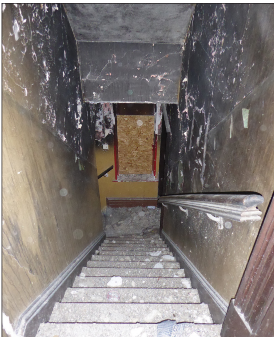
Figure 49: View of archway bridge staircase from second floor (© Historic England, photograph: Alastair Coey Architects 2019)
