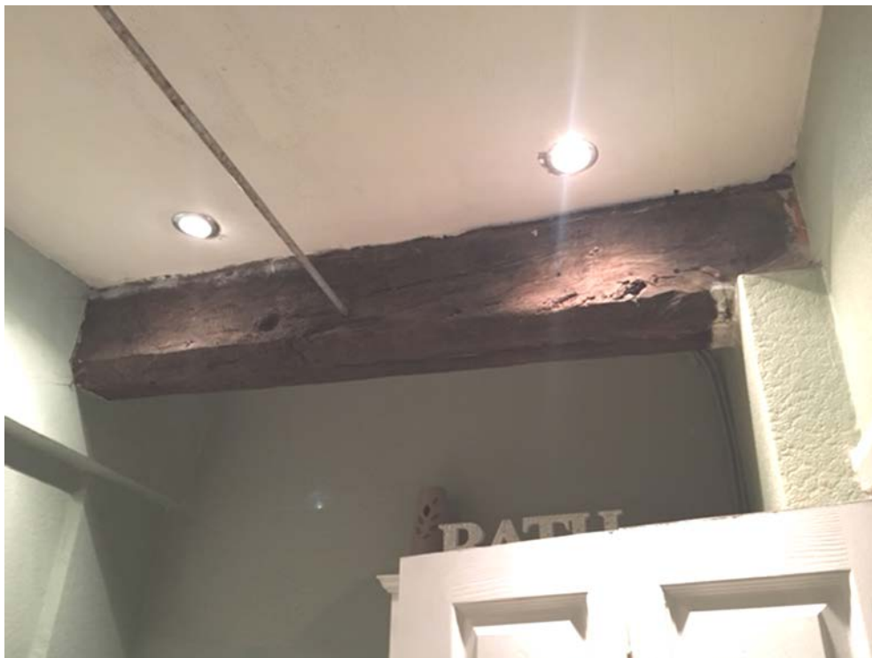
Figure 11: Cross-wing - north-south first floor beams, visible on the ground floor, photograph taken from the west (Alison Arnold)
