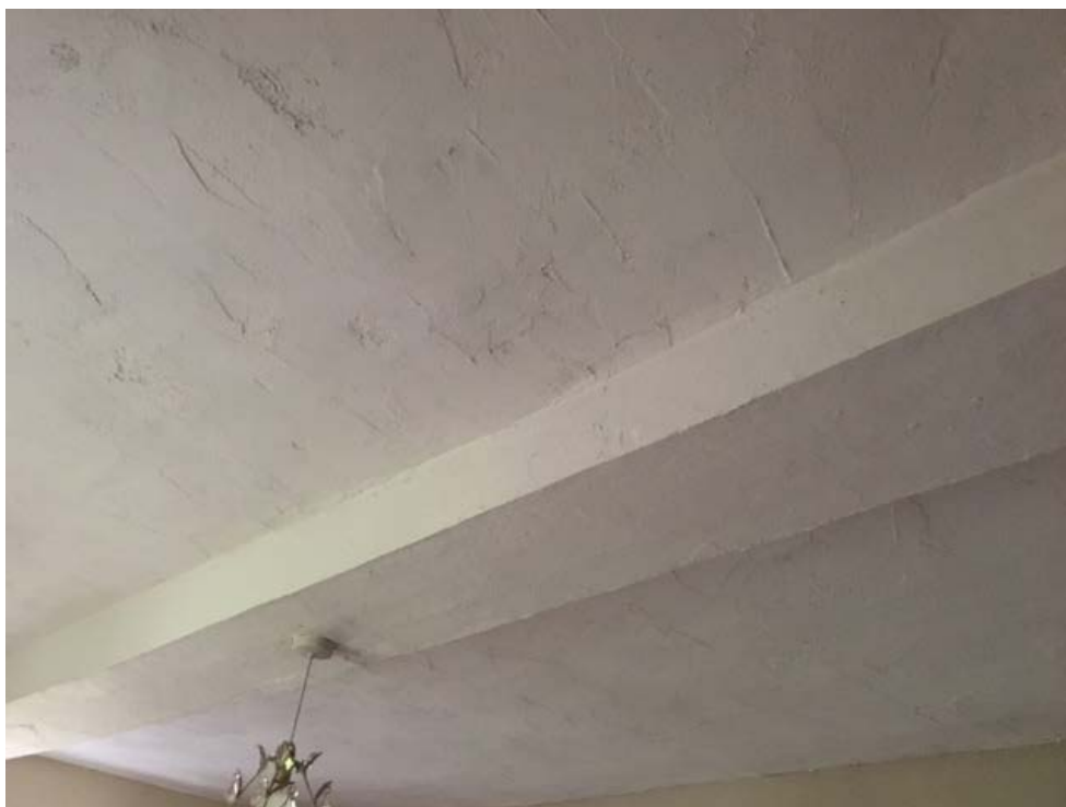
Figure 12: Cross-wing - east-west first-floor beam, visible from the ground floor, photograph taken from the south-east (Alison Arnold)
