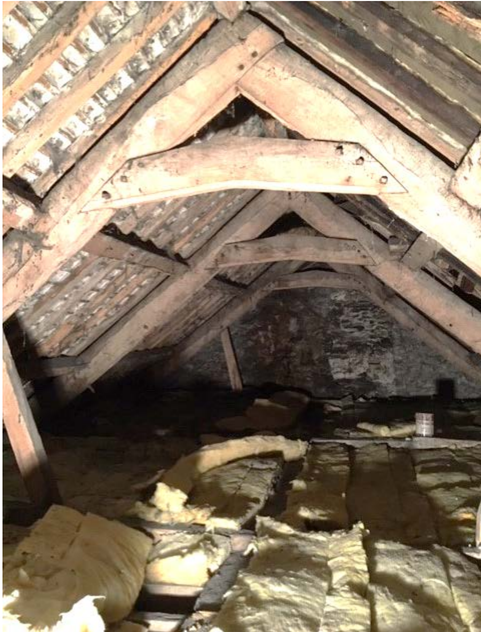
Figure 5: Hall roof, with truss 3 in the foreground, photograph taken from the south (Alison Arnold)
