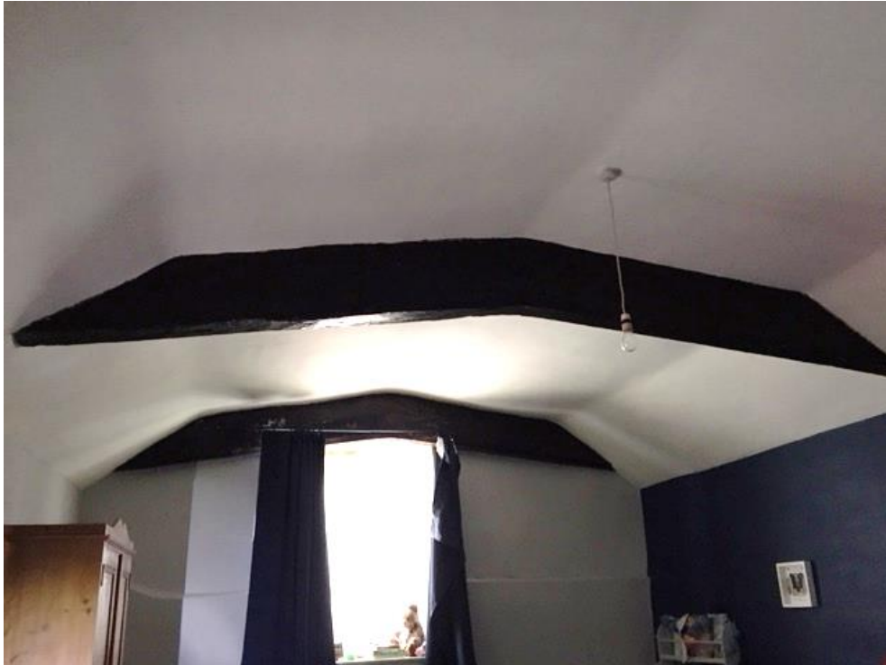
Figure 8: Cross-wing - the tiebeams of trusses 1 and 2, photograph taken from the west (Alison Arnold)
