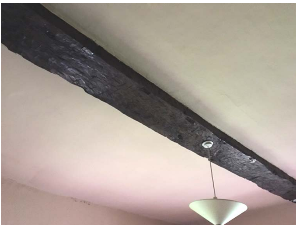
Figure 13: Cross-wing - second-floor beam, visible from the first floor, photograph taken from the east (Alison Arnold)
