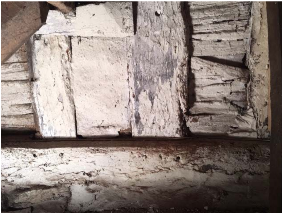
Figure 7: Hall - partition between the lounge and stairs, photograph taken from the south (Alison Arnold)
