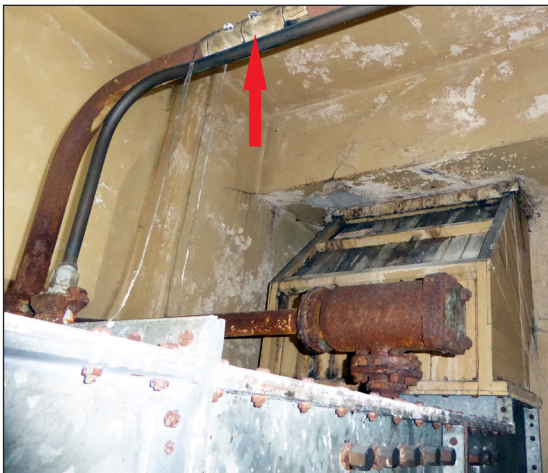
Figure 36: Intake duct to evaporator with liquid separator (© Historic England, photograph: Alastair Coey Architects 2019)
