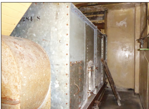
Figure 35: Room GF1B showing the fan, evaporator, and expansion valve (© Historic England, photograph: Alastair Coey Architects 2019)
