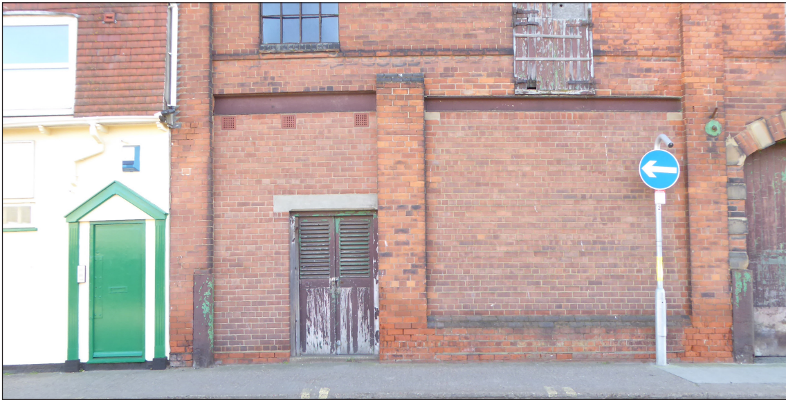
Figure 15: Infilling of a previous entrance to the west elevation (© Historic England, photograph: Alastair Coey Architects 2019)
