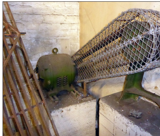
Figure 37: Fan motor (© Historic England, photograph: Alastair Coey Architects 2019)
