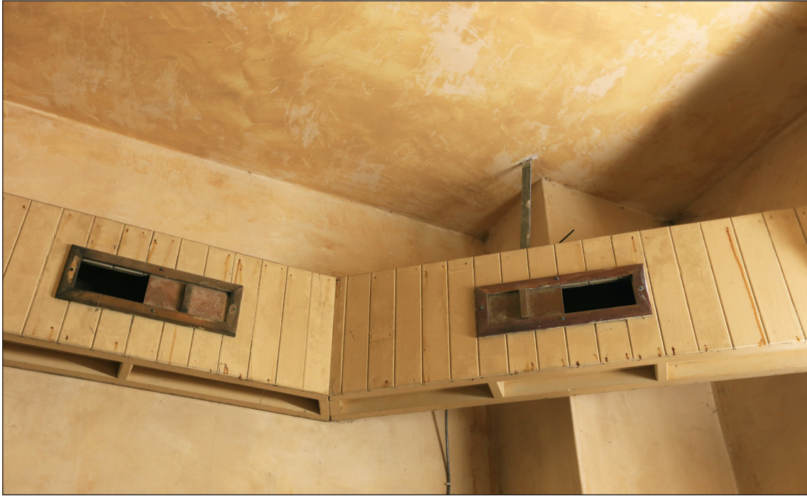
Figure 40: Adjustable openings in chilled air duct (© Historic England, photograph: Alastair Coey Architects 2019)
