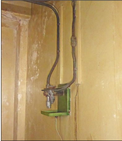
Figure 38: Expansion valve (© Historic England, photograph: Alastair Coey Architects 2019)
