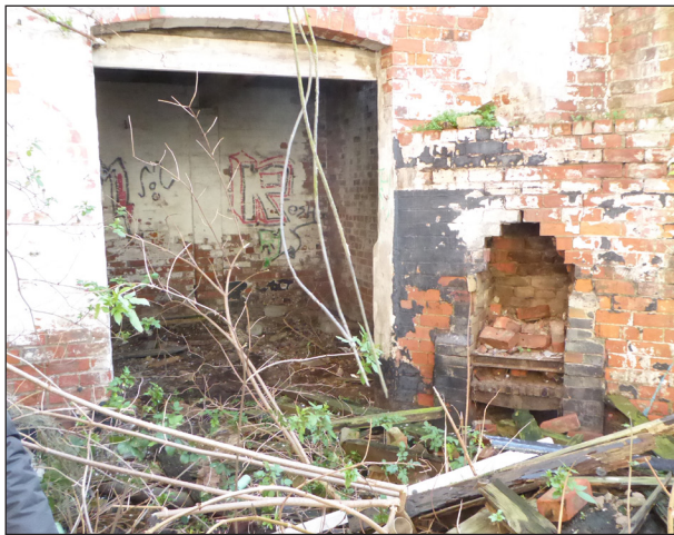
Figure 19: Surviving features of fireplace to coopers’ store (© Historic England, photograph: Alastair Coey Architects 2019)
