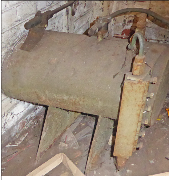
Figure 33: Receiver (© Historic England, photograph: Alastair Coey Architects 2019)
