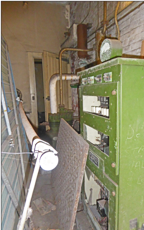
Figure 27: Looking east along Room GF1A with compressor seen on the right-hand side (© Historic England, photograph: Alastair Coey Architects 2019)
