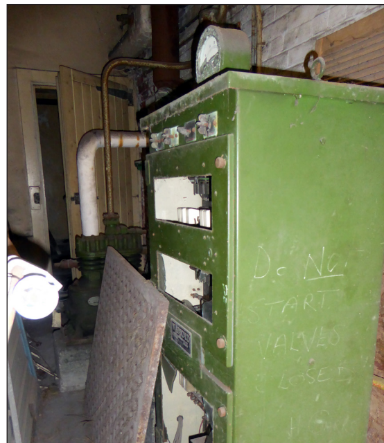
Figure 30: Motor control cabinet (© Historic England, photograph: Alastair Coey Architects 2019)
