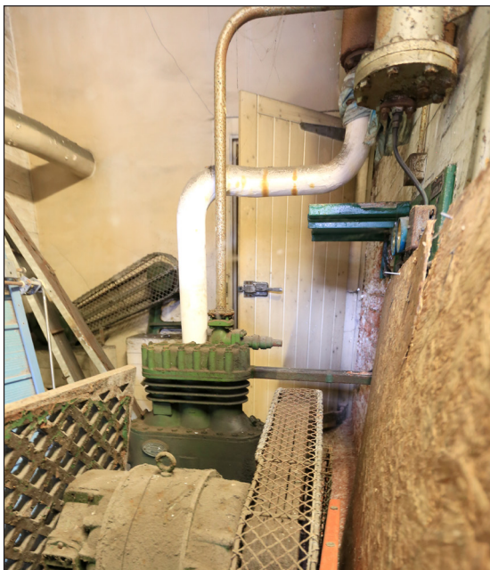
Figure 29: Vee-belt drive from motor to compressor (© Historic England, photograph: Alastair Coey Architects 2019)
