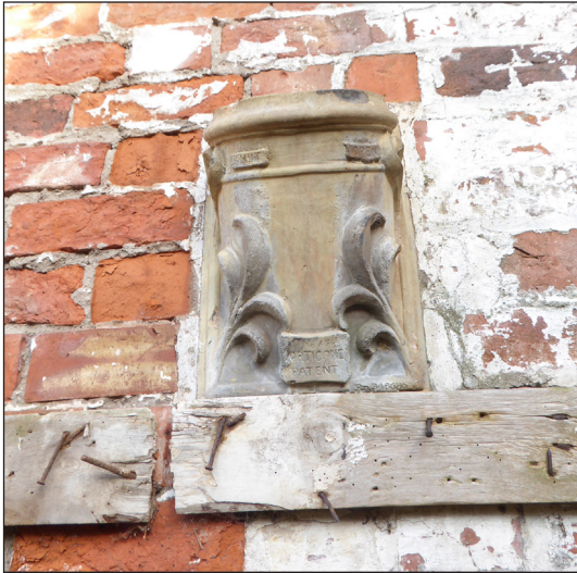
Figure 20: Surviving terracotta air vents in the coopers' store (© Historic England, photograph: Alastair Coey Architects 2019)
