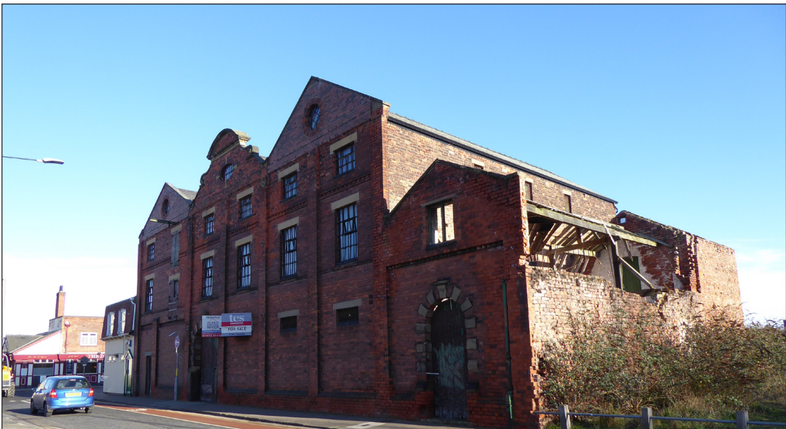
Figure 16: View of warehouse building as seen from East Street (© Historic England, photograph: Alastair Coey Architects 2019)
