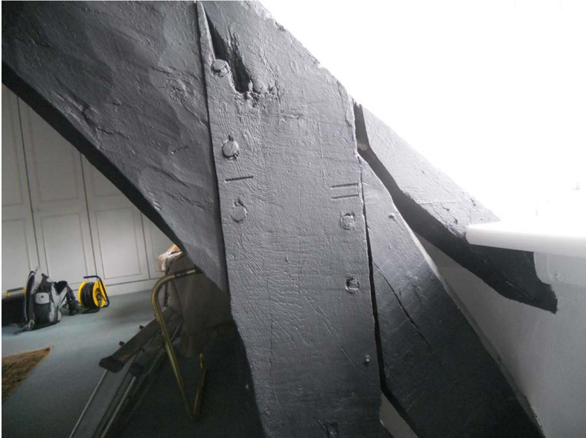
Figure 3: View of the post supporting the east rafter of the south truss of the front range, which produced samples cn9wst05a–b (photograph Martin Bridge)
