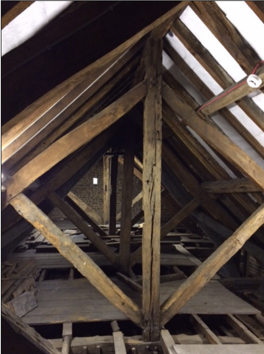
Figure 5: Courtroom roof, truss 2 in foreground, photograph taken from the east (Alison Arnold)
