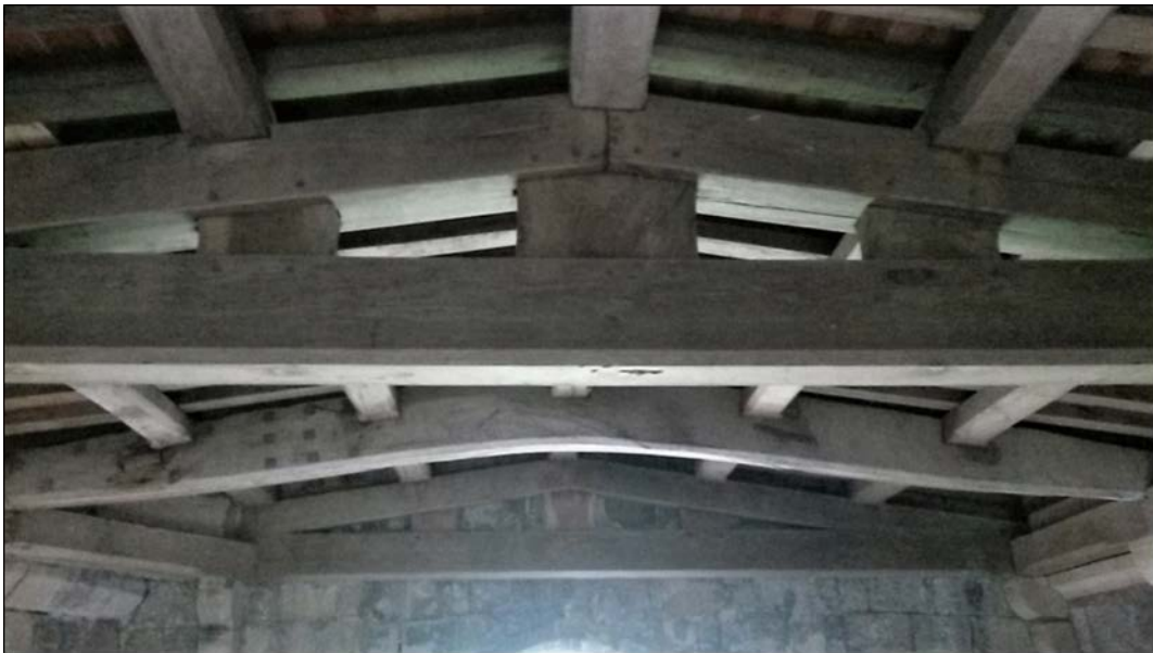
Figure 5: Castle tower; roof, truss 5 in foreground, photograph taken from the north (Alison Arnold)
