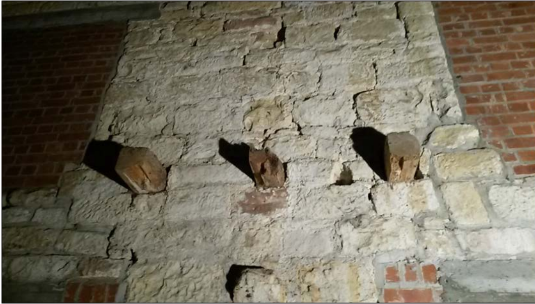
Figure 10: Stable block; remnants of floor joists, photograph taken from the west (Alison Arnold)
