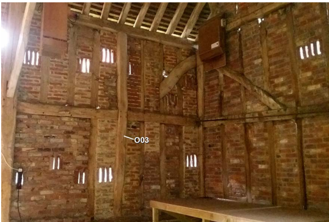
Figure 5: Interior of the barn showing the south-east corner with the location of sample buny003, from the intermediate storey post in the southern bay (photograph: Martin Bridge)
