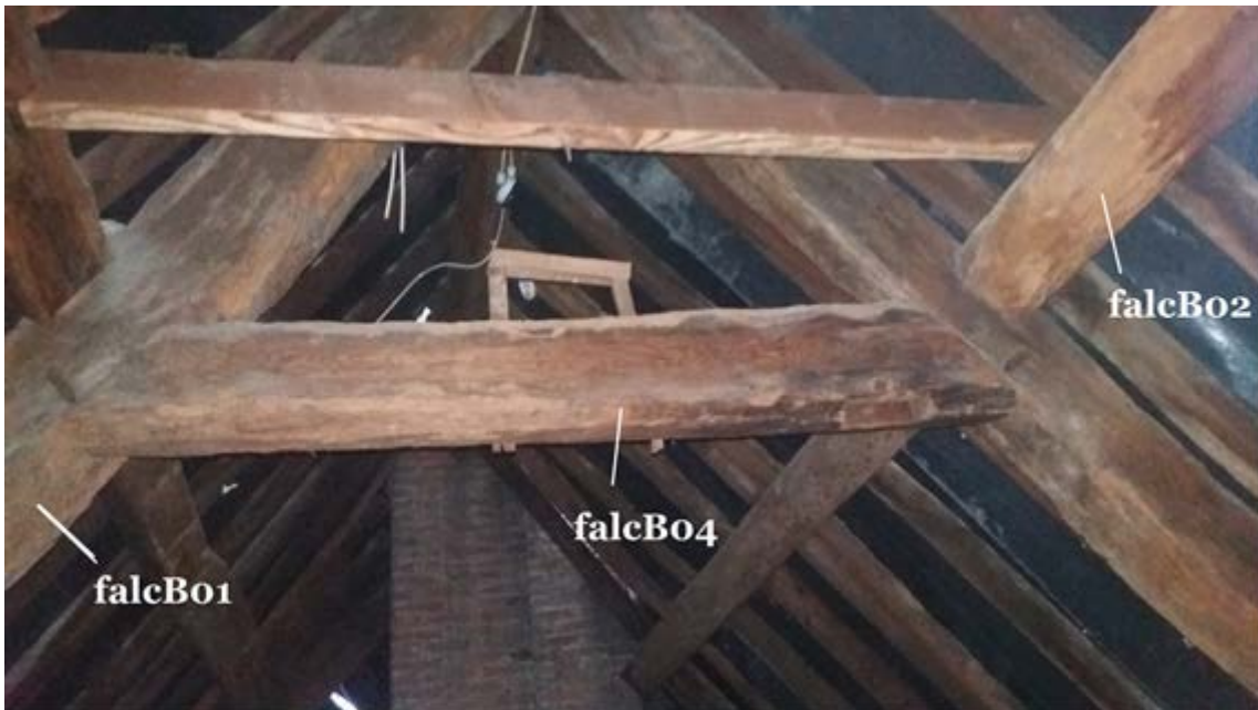
Figure 4: View looking west from the entry into the elm roof, showing truss 2 and the stack behind, with some of the timbers sampled (photograph Martin Bridge)
