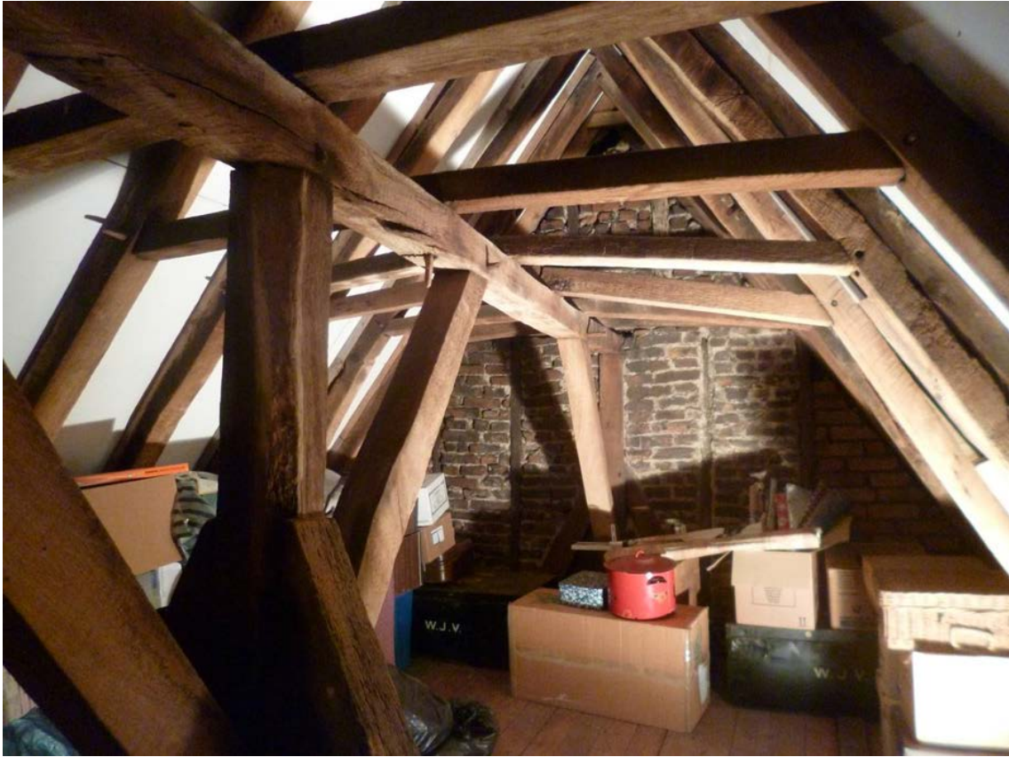
Figure 5: 19 Ladygate, photograph of the roof with truss 5 in the foreground, photograph taken from the south (Alison Arnold)
