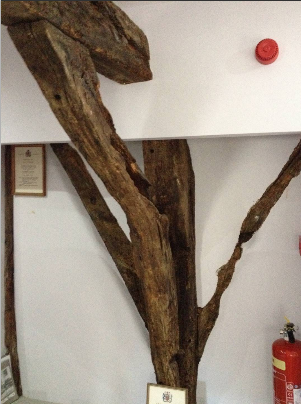
Figure 5: The west post of truss V, photograph taken from the north-east (Alison Arnold)
