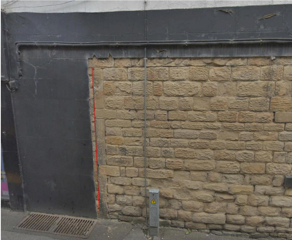
Figure 31: Blocked-up doorway to west-facing facade of 63 Daisy Hill, potentially the original entrance (indicated in red)
