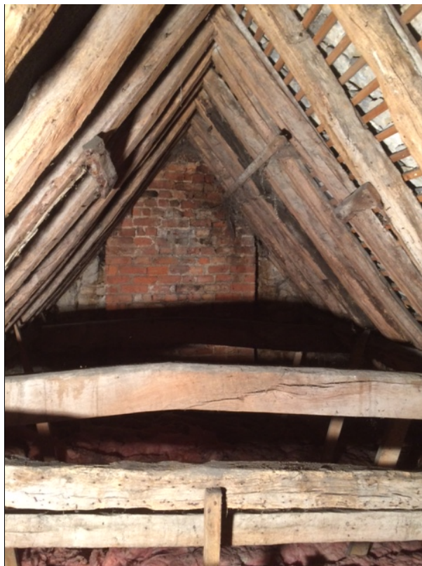
Figure 5: Cross-wing roof, photograph taken from the north, the collar of frame 27 centre (photograph Alison Arnold)
