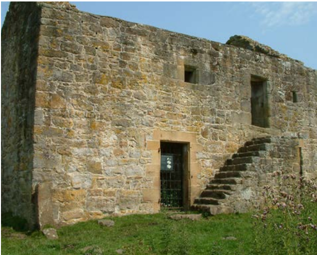
Bastles. Black Midden is an isolated, 15th- or 16th-century bastle set in an elevated position above Tarsset Burn, east of Kielder Forest. The byre entrance, square headed with a narrow chamfer to the lintel, is set in the east gable. The entrance on the front elevation is secondary. The domestic area at first floor level is reached by an external stone stair on the front elevation. The doorway is square headed, with narrow, continuous chamfer to lintel and jambs. Sockets under the lintel are possibly for vertical bars. Sockets are evident for a harr hung door and a draw bar. Photo © Jen Deadman
