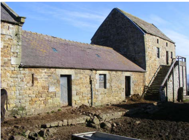
Some of the more accessible bastles, as here to the north of Bellingham, were incorporated within farmsteads that were extended and remodelled as part of the 19th-century agricultural improvements across the area. The upper floor of this bastle was used as a granary, as part of a courtyard group set within a landscape transformed through regular enclosure. Photo © Jen Deadman
