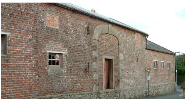
This early 19th-century brick barn, with sandstone dressings set on a cobble plinth, is distinctive of the area. From the 18th century onwards, many farmsteads were constructed of sandstone or locally made bricks. There was a good deal of transport of sandstone dressings into adjacent districts and use of such dressings with brickwork. The distinctive flat arch with voussoirs and keystone is frequently found on combination barns which do not have the projecting porch. Photo © Jen Deadman
