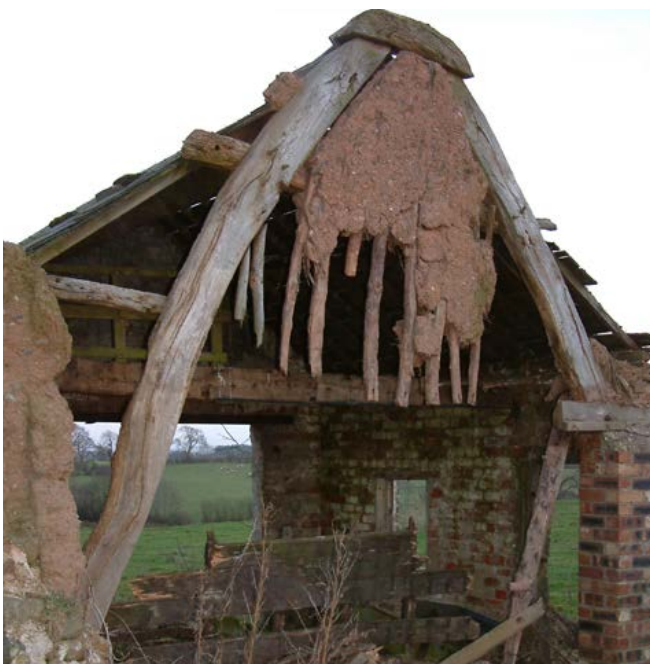
A very rare surviving example of a cruck-framed field barn with remnants of clay walling. Photo © Jen Deadman
