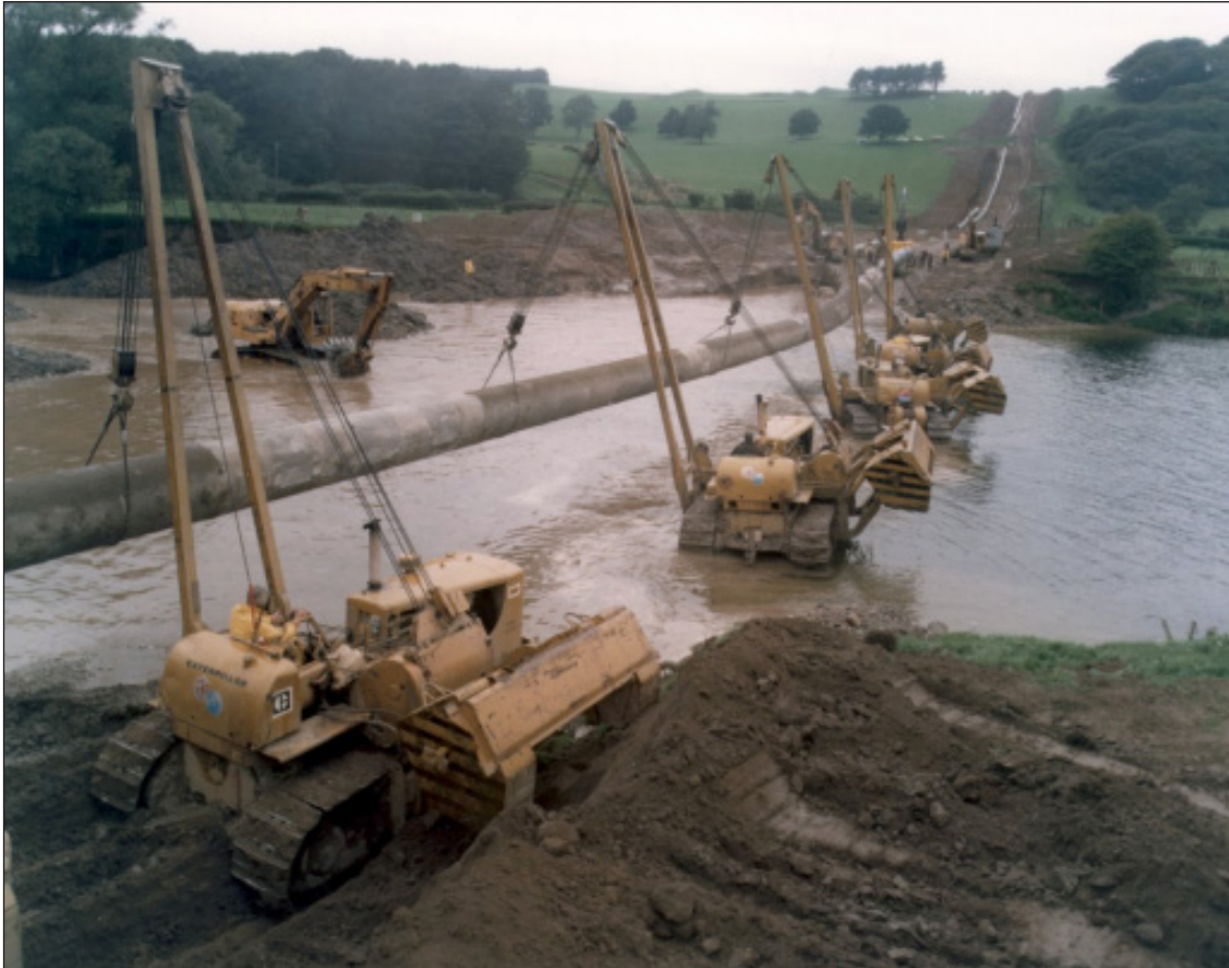
Figure 2.66. Building the National Gas Transmission System, Laying a transmission pipeline across a River. Source National Grid Gas Archive.
