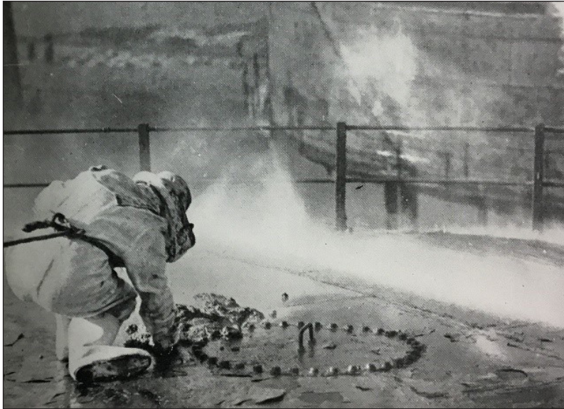
Figure 2.58 (Left) Engineers attempting to repair a burning gasholder, Romford, Essex during the Second World War. Source National Grid Gas Archive.
