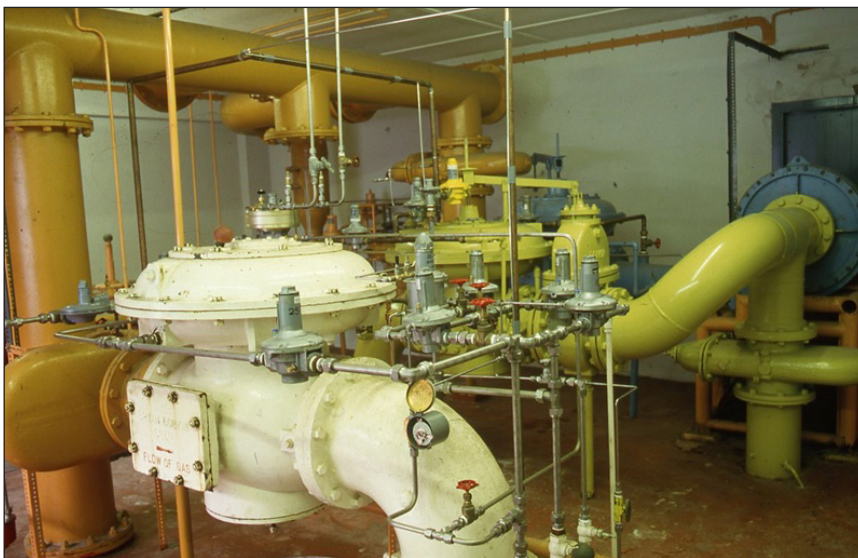
Figure 3.95 Inside a large governor house, Cornwall, 1980's. Image courtesy of IGEM archive.
