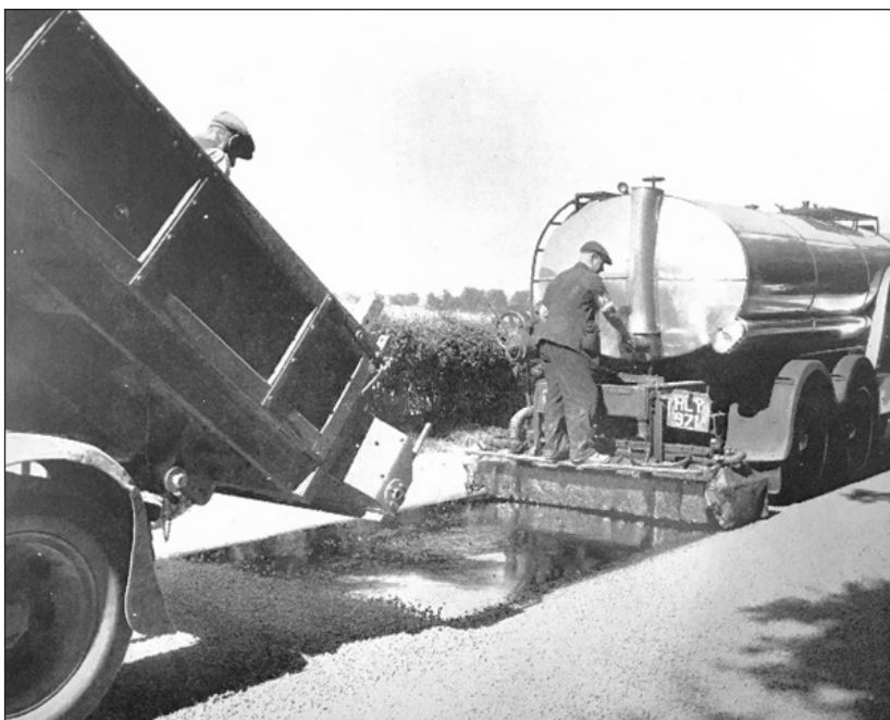
Figure 3.195 Laying coal tar pitch as tar Macadam. Image courtesy of National Grid Gas Archive.
