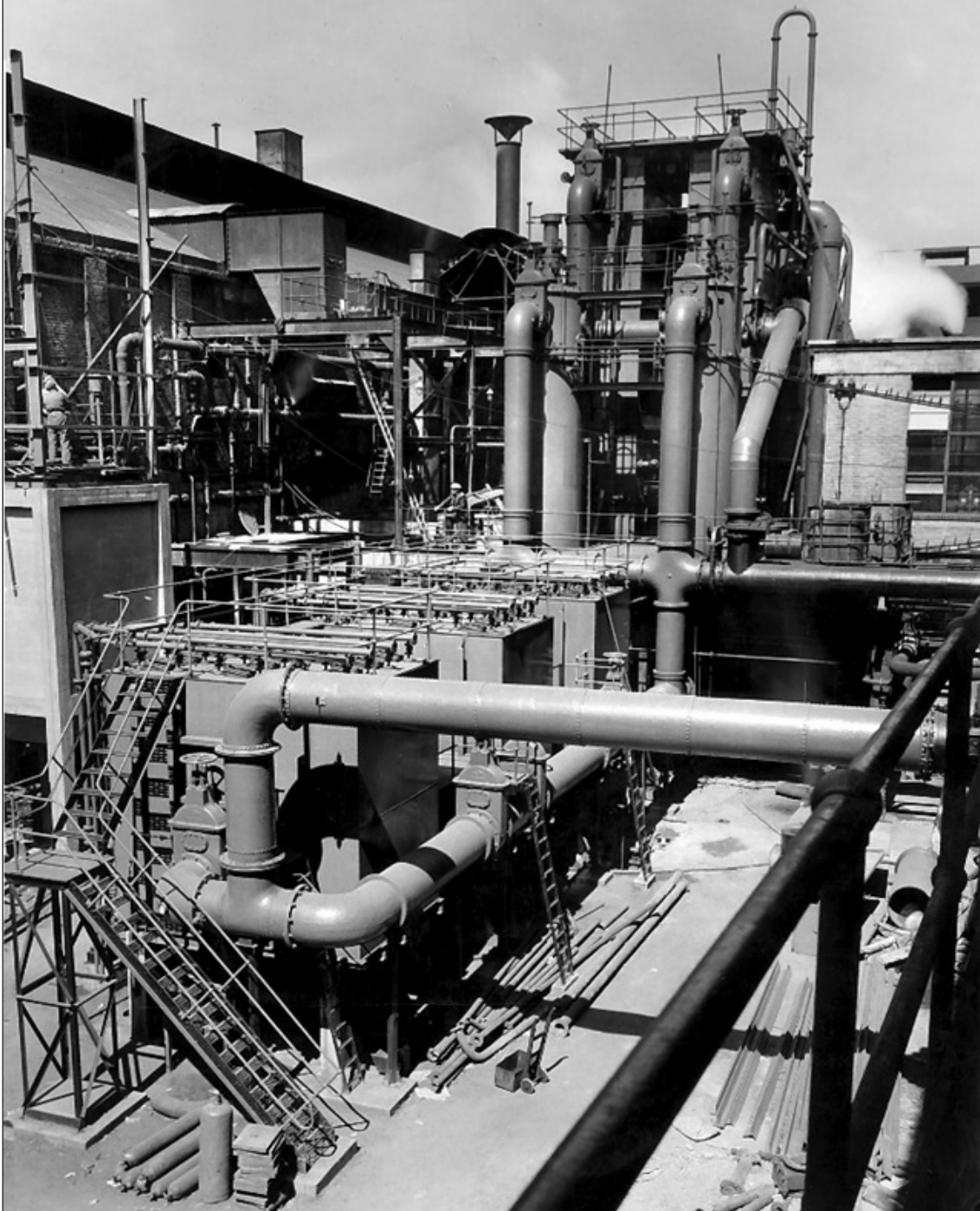
Figure 3.70 Ammonia washers with electrostatic detarrers and primary and secondary condensers in the background, Rotherhithe gasworks, London 1948. Image courtesy of National Grid Gas Archive.
