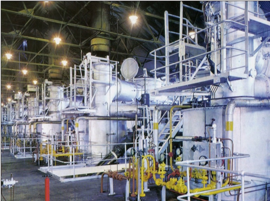
Figure 3.120 The interior of the water gas plant building at the former East Greenwich gasworks. Image courtesy of National Grid Gas Archive.
