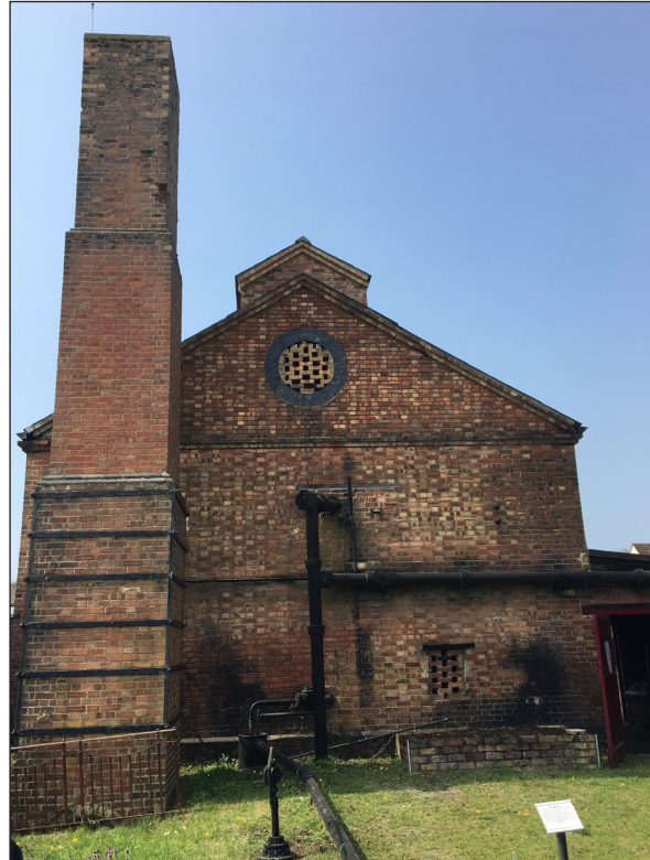
Figure 3.5 The surviving horizontal retort house, showing the chimney and louvered roof, Fakenham gasworks 2018. Source R. Thomas.
