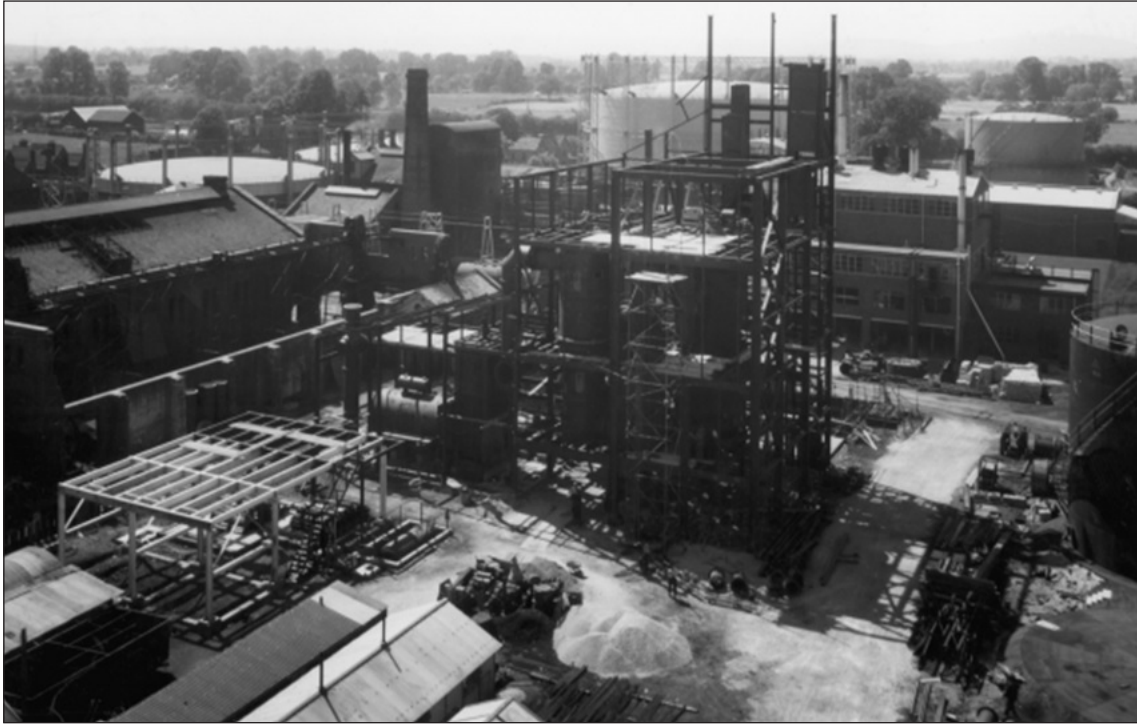
Figure 3.149 The Hempsted Gasworks Gloucester, where a range of oil gasification processes were operated, including the Hall, Jones, Koppers-Hasche and Gas Integrale processes. Image courtesy of National Grid Gas Archive.
