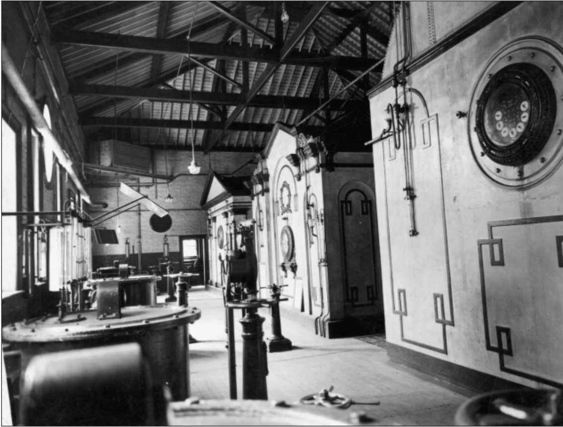
Figure 3.98 Three station meters in the meter house. Image courtesy of National Grid Gas Archive.
