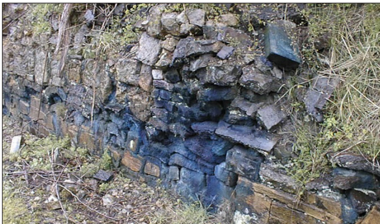
Figure 3.81 Blue staining on a wall at a former gasworks from Spent Oxide. Source R. Thomas.
