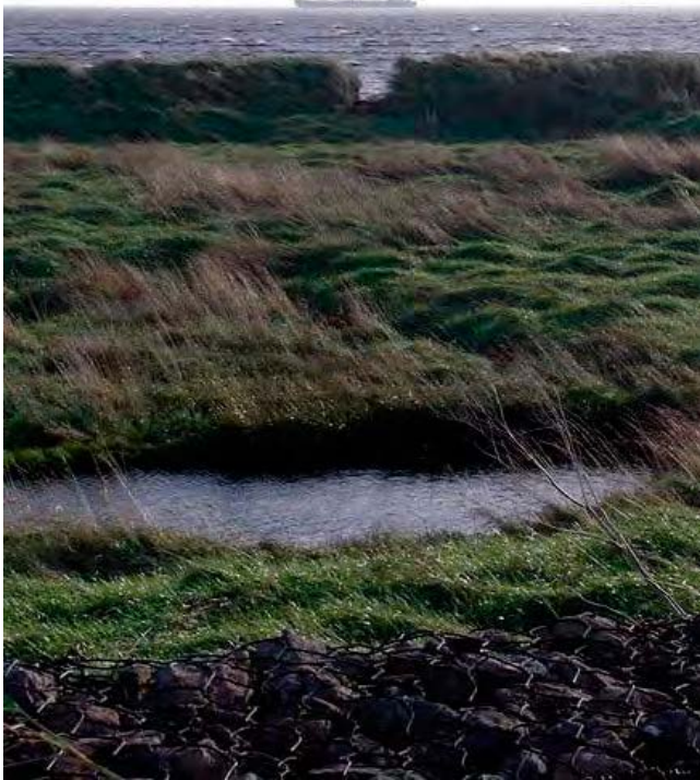
Damaged floodbank and shipping, Sunk Island. © Paul Glazzard
