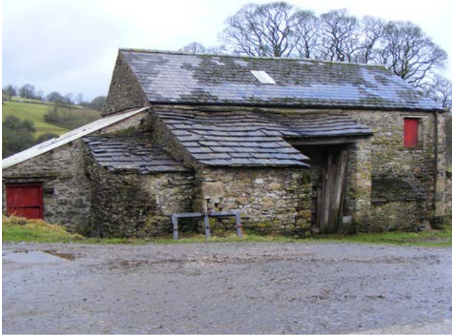
This bank barn on a steading close to the river Lune is set into the hillside on three levels. It contains, in one structure, all the traditional working functions of the farmstead. The threshing barn, which fronts the main range at right angles, has the standard arrangement for a bank barn of hay mew to the left with shippon at a lower level to the right, above which is a loft area. Photo © Jen Deadman
