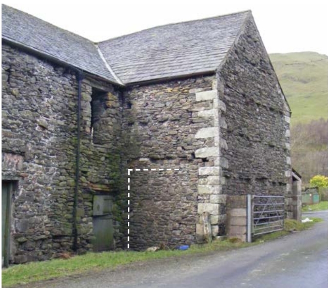
Blocked cart entry at lower level of ramped barn. Photo © Jen Deadman
