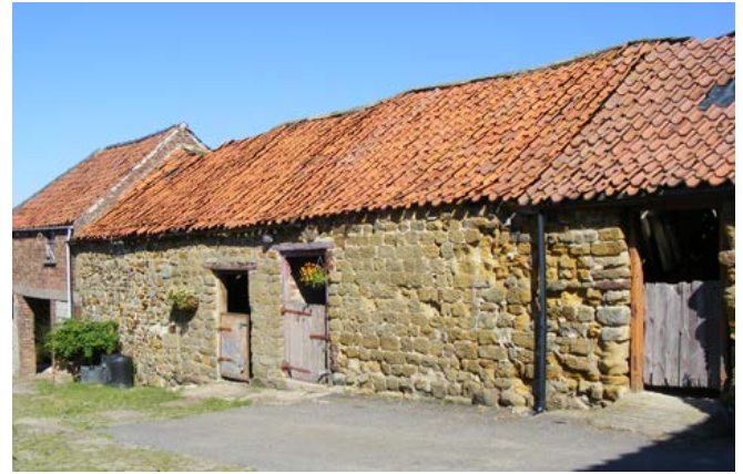
Four bay, cruck-framed, single-storey, multifunctional range with an early 20th-century cart shed and granary adjoining The range comprises threshing barn with two byres and a cart shed set under one roofline. To the rear behind the threshing barn is a horse engine house, now ruinous. The position of the drive shaft can be located on the rear wall of the barn. Photo © Jen Deadman
