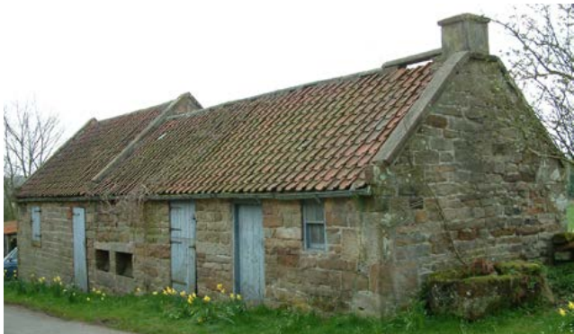
Stables A small stable adjoining a pigsty, the stack indicating the position of a meal house for boiling feed. Photo © Jen Deadman
