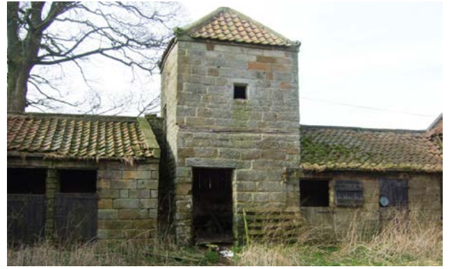
Little Fryup Dale. Dovecote taking the form of tower over former archway set between two single-storey ranges in an estate farmstead rebuilt c 1850 to a regular multi-yard plan. Photo © North Yorkshire Moors National Park
