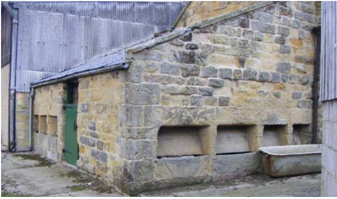
The scale of pigsties, particularly in the eastern part of the area (as here at Hackness), is comparable to that of areas further to the south, particularly the Vale of Pickering and Holderness. This large pigsty has feeding troughs built into both side walls. It is adjacent to a mill. Photo © Jen Deadman
