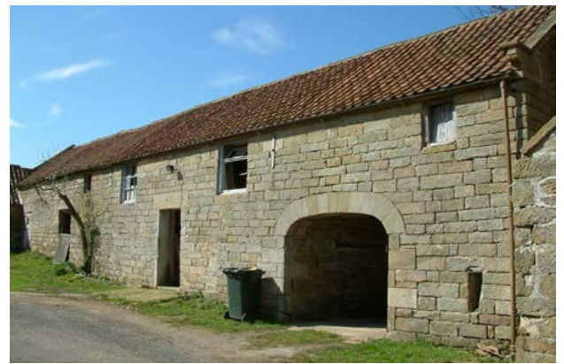
Here the granary is sited over a cart shed and stables, and accessed by external steps in the gable end. Photo © Jen Deadman
