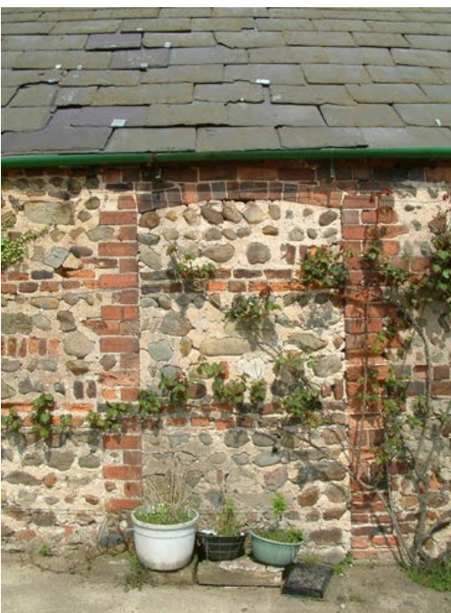
Courses of brickwork help maintain stability in random cobble walls. Brick is used also as quoins and as dressings to openings. Photo © Jen Deadman
