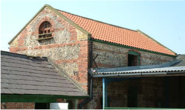
The decorative use of brick quoins and lacing to this mid-19th-century combination barn is enhanced by the arched recess with doveholes in its gable end. Photo © Jen Deadman
