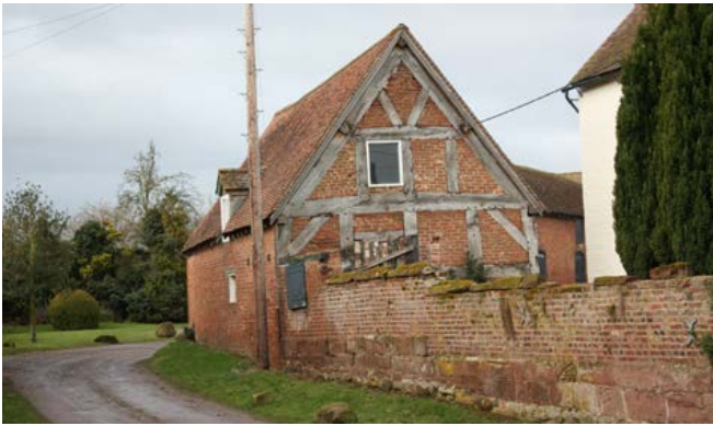
Across the area, particularly in Shropshire, timber-framed barns were often encased in brick – here the gable end was left exposed but often the framing is completely hidden externally. Photo © Bob Edwards
