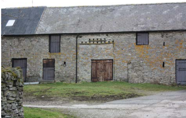
The majority of barns are stone built and incorporated into combination ranges. The threshing door was blocked (and given pigeon holes) in the late 19th century when additional doors were inserted for its conversion to a cow house and stables. Photo © Bob Edwards
