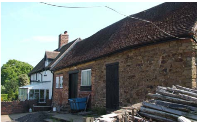
In the southern part of the area around the Wyre Forest, smaller farmsteads and smallholdings including linear plans are intermixed with medium-scale farms. This linear farmstead is the product of development over time with buildings added to the gable end of the farmhouse. Photo © Worcestershire County Council
