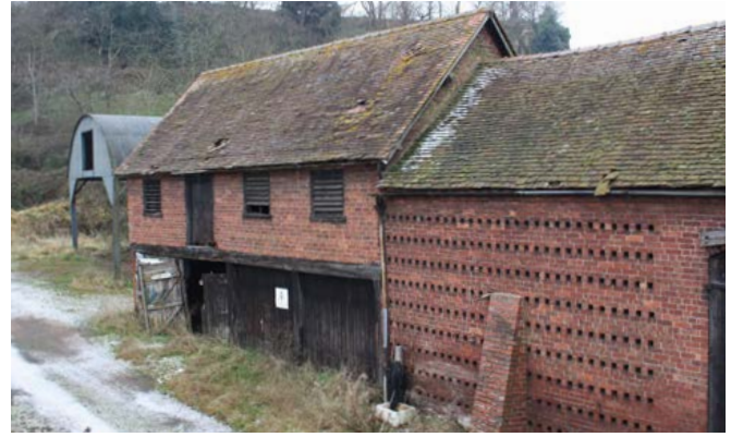
Forming part of a regular U-plan range, the granary is located next to the barn and above an outward-facing cart shed. Large combined cart shed and granary ranges are typical of the large, arable-based farmsteads of the area, some dating from the mid- to late 18th century. Photo © Bob Edwards
