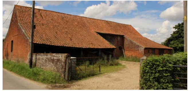
Outshots for housing cattle added to a 17th-century barn at Runhall. Photo © Bob Edwards
