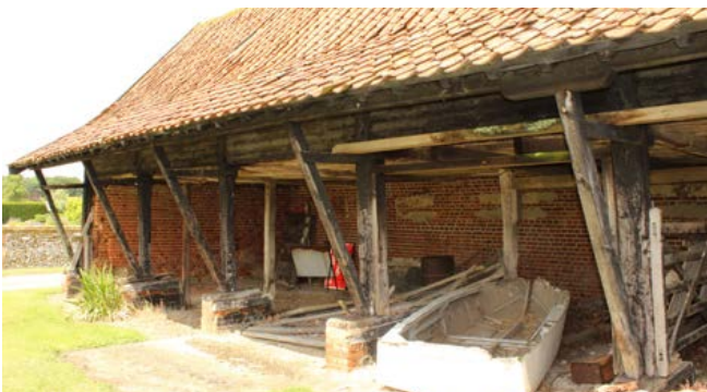
Mid-19th-century cart shed with unusual use of raked timbers to support projecting roof. Photo © Bob Edwards
