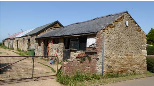
Early to mid-19th-century cow houses and loose boxes at Gayton. Photo © Jeremy Lake
