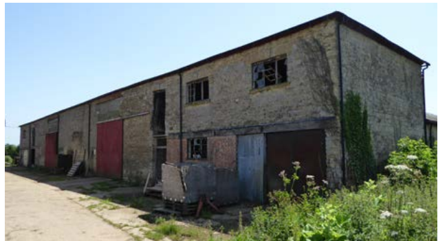
A large, mid-19th-century combination barn, with two threshing floors and a granary sited over a cart shed. This arrangement, with a combination barn sited to one side of a cattle yard, is found in the larger farmsteads established from the late 18th century. Photo © Jeremy Lake
