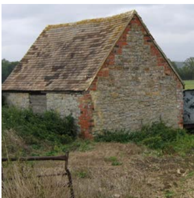
A small field barn for cattle, of a type found in areas, as seen here, of large-scale, regular enclosure where large farms required structures sited away from the main stabling. Photo © Jeremy Lake
