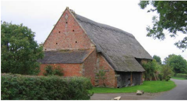
A very rare surviving example – for this area in particular – of a large 16th or 17th-century barn, originally timber-framed, on the edge of a village in the Feldon area. Its scale testifies to the development of a prosperous class of Feldon farmers by this period, and has enabled the building to be adapted and used through the changes of the 19th and 20th centuries. Early barns are concentrated to the south of the area, close to the Cotswolds and the Severn and Avon Vales. Photo © Jeremy Lake
