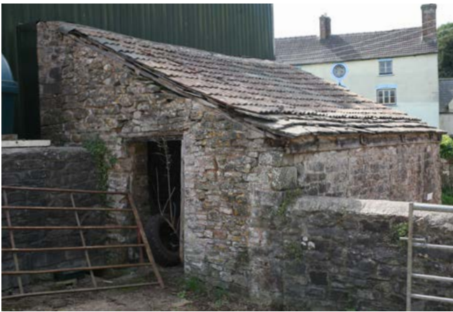
Pigsty with monopitch roof. Pigsties were the most common type of building to remain on smallholdings, and were built in large numbers in this area in the 19th century. Photo © Sam Hale
