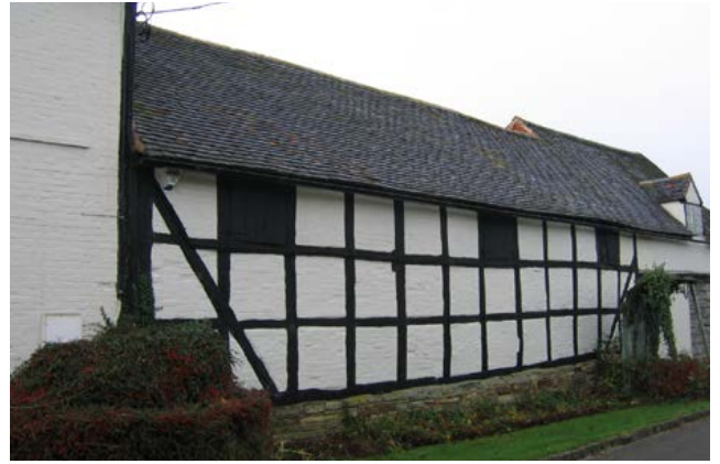
A rare, surviving example of a timber-framed cow house or stable. Buildings such as this in timber frame are very rare, and otherwise are concentrated in the wood pasture landscapes of East Anglia, the Weald of Kent and Sussex and to the west of the West Midlands region. Photo © Jeremy Lake
