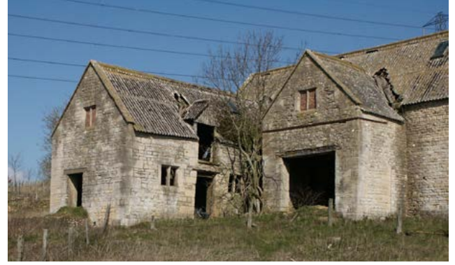
Another typical arrangement, on a farmstead that served fields enclosed in the 15th century on the eastern edge of Cleeve Hill, with a stable range extending from the barn and a small granary incorporated in the barn porch. Photo © Jeremy Lake
