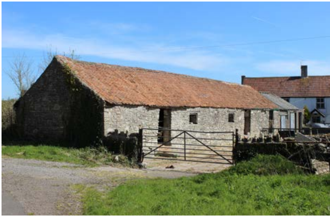
A single-storey, mid-19th-century cow house for housing dairy cattle. Photo © Bob Edwards
