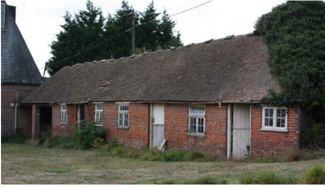
This single storey stable range is of early 19th-century date but with possible earlier foundations.
