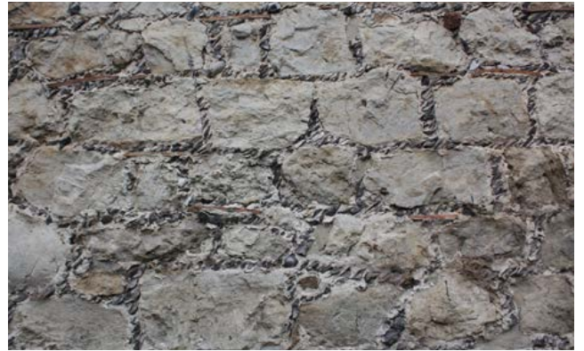
The insertion of small stones into the mortar joints of stone walls (a technique known as galleting) can occasionally be found in the North Downs. Here, small pieces of flint have been used. Photo © Bob Edwards
