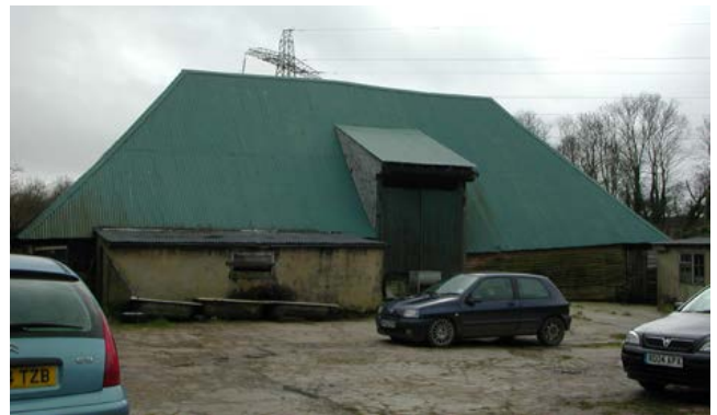
An aisled, timber-framed threshing barn of five bays, aisled to all sides. Photo © Bob Edwards
