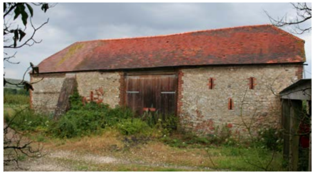
The local sandstone was widely used for farm buildings in the 18th and 19th centuries, typically with brick quoins and dressings. Photo © Bob Edwards
