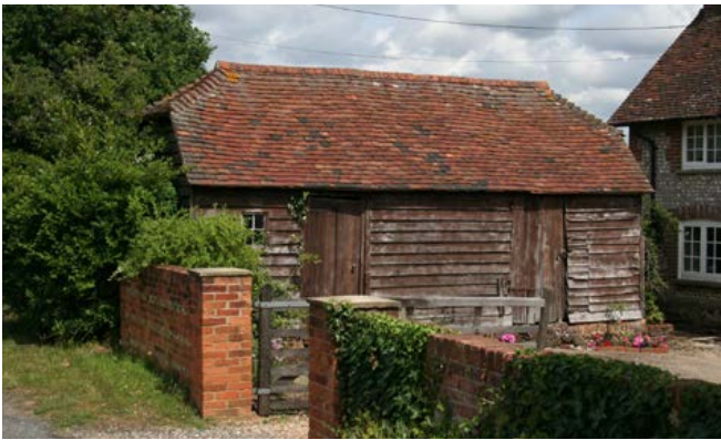
A small, timber-framed stable, typical of some of the smaller farmsteads of the Greensand. Photo © Bob Edwards
