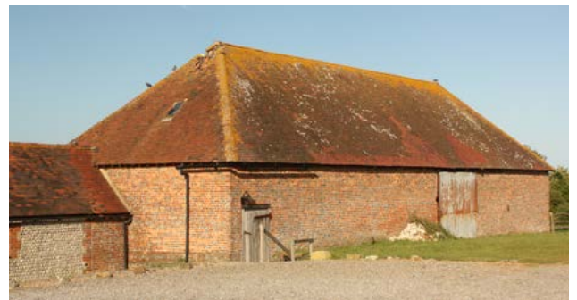
A rare survival of an 18th-century, brick-built barn with a hipped roof. The single door possibly indicates the presence of animal housing in one end. Photo © Bob Edwards
