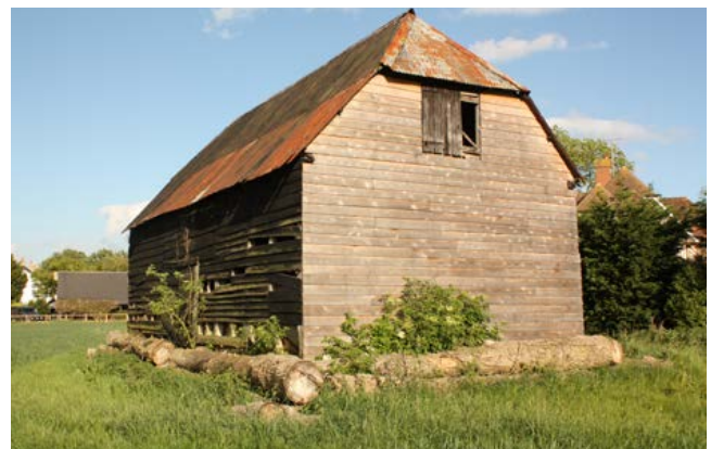
The tree trunks around this building obscure the fact that it stands on staddle stones. It is uncertain whether this was a staddle barn or a very large granary. A tie beam bears the date 1724, which would suggest it was a granary, as most staddle barns were built in the decades around 1800. Photo © Bob Edwards
