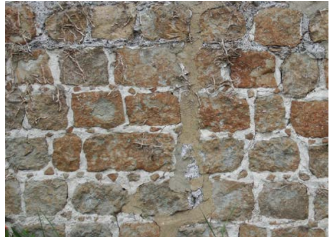
Galleting is the insertion of small pieces of stone into the mortar joints, here done for decorative effect. Although not common, galleting is a highly distinctive feature of the area. Photo © Bob Edwards
