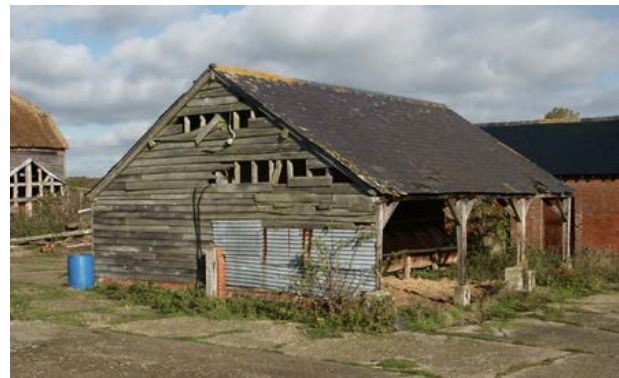
Cattle housing typically takes the form of open-fronted shelter sheds ranged around the yard. This rare example has two three-bay sheds set back-to-back serving two adjoining yard areas. Inside, mangers formed from elm planks survive, together with evidence that cattle were tethered in these sheds. Photo © Bob Edwards
