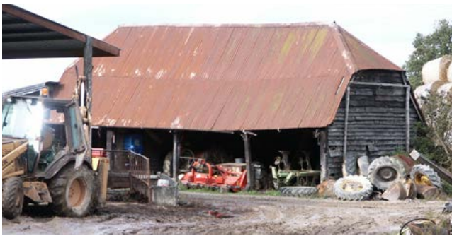
Cart sheds were common to most farmsteads, typically located alongside a track leading into the farmstead. These buildings have been vulnerable to loss and are rarely listed. Photo © Bob Edwards
