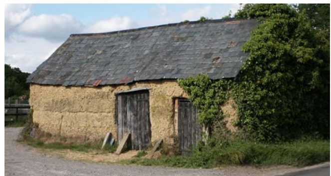
A small, earth-built, stable or cow shed, typical of the small-scale farm buildings that would have been seen on many New Forest small-holdings. Such survivals are now very rare. Photo © Bob Edwards
