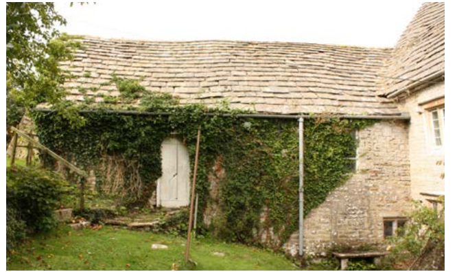
This range, attached to the 17th-century and earlier Dunshay Manor house, was constructed, or possibly remodelled, in the 19th century to form a cider house with a cellar at the lower level and an upper floor access by the door to the left. Photo © Bob Edwards
