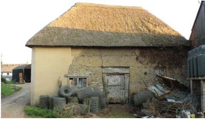
This earth-walled stable or cow house is a rare surviving example of the use of cob in the area, possibly reflecting the once more widespread use of earth for the construction of farm buildings which have been replaced by stone in the later 18th and 19th centuries. Photo © Bob Edwards
