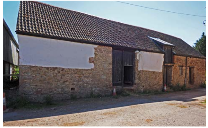
Straight joints, other evidence of phasing and the presence of render as here, on this threshing barn and attached stable can indicate how buildings have gradually been rebuilt or extended in stone or brick from earlier cob-walled buildings. Photo © Eric Berry
