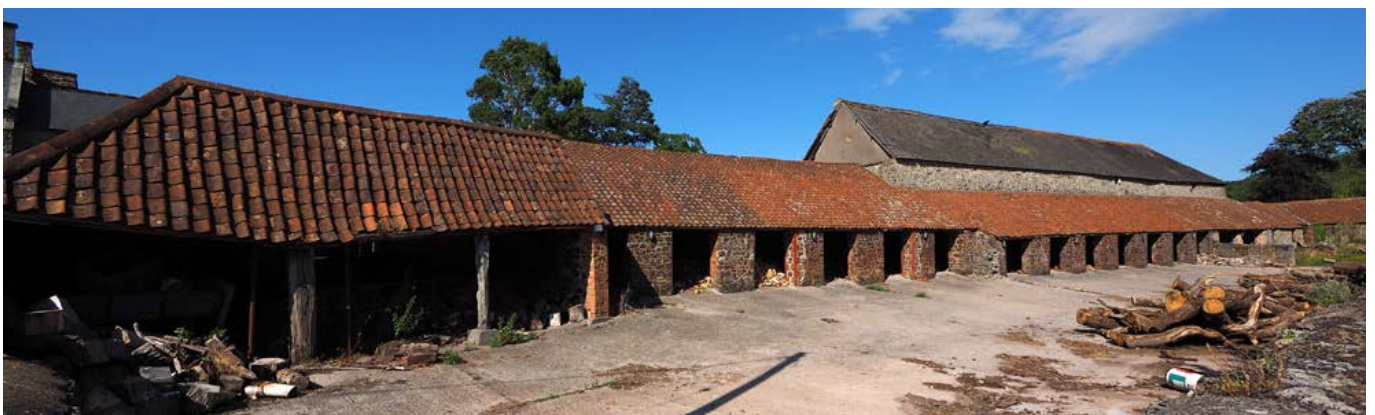
The shelter sheds attached to the tithe barn at East Quantoxhead (see page 3). Photo © Eric Berry
