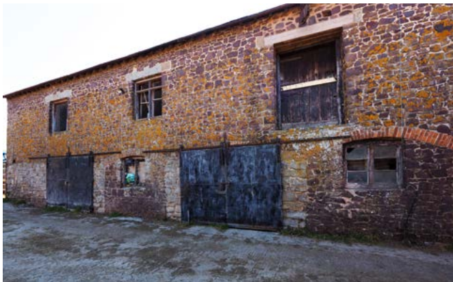
A large, mid-19th-century bank barn with ground-floor cattle housing, on the north Somerset coast. Photo © Eric Berry
