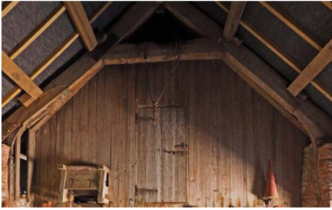
Jointed crucks – marked here by the pegs driven into the jointing of the lower curved section of crucks and the main rafters – are a distinctive feature of this area and areas extending to the south and west. Photo © Eric Berry
