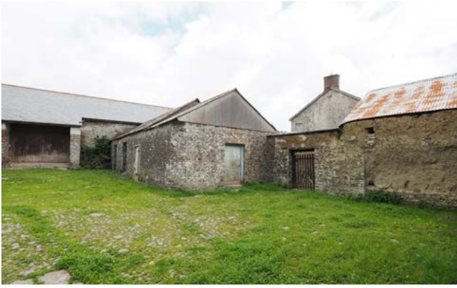
A threshing barn (left), attached cow house and a cob-walled farm buildings at Sutcombe. Photo © Eric Berry
