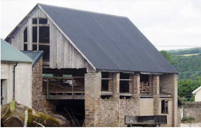
A mid-19th-century linhay, formerly open-fronted and walled-in as part of the move from fatstock which favoured sheds facing yards to dairy cattle which were stalled in cow houses. Photo © Eric Berry
