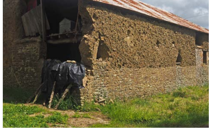
Cob walling to a barn, with ventilation holes formed by slates. Photo © Eric Berry
