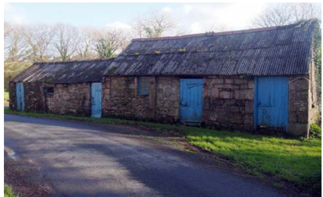
Vellanewson. Roofing is more likely to be corrugated iron, tin or asbestos than any other material now, notwithstanding historic use of slate and thatch. Photo © E Berry.
