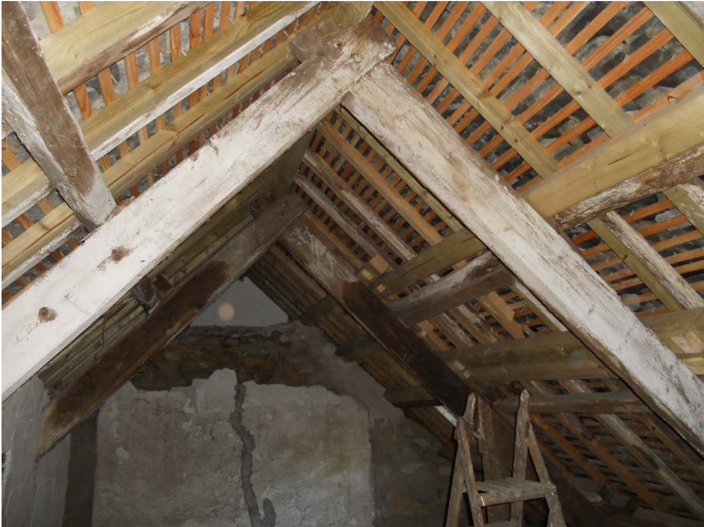
Figure 3: View of the roof, looking west, showing small scantling conifer timbers (photograph Martin Bridge)
